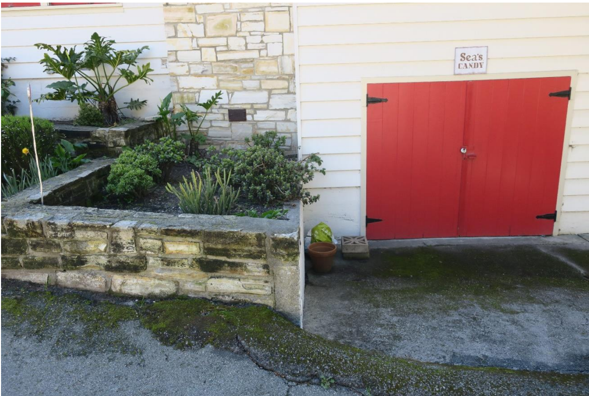
Planter-style retaining wall east of and adjacent to the driveway fronting 1 st Avenue. View south.
