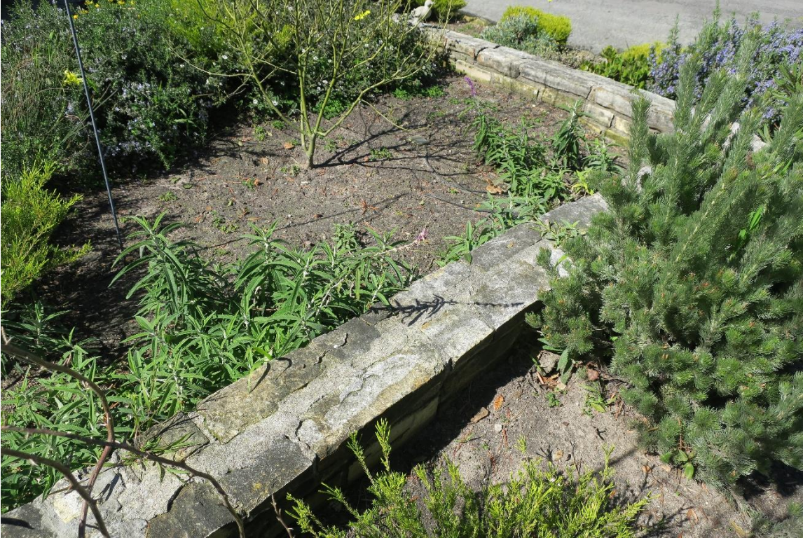
Retaining/garden wall just outside the east and north property lines.
