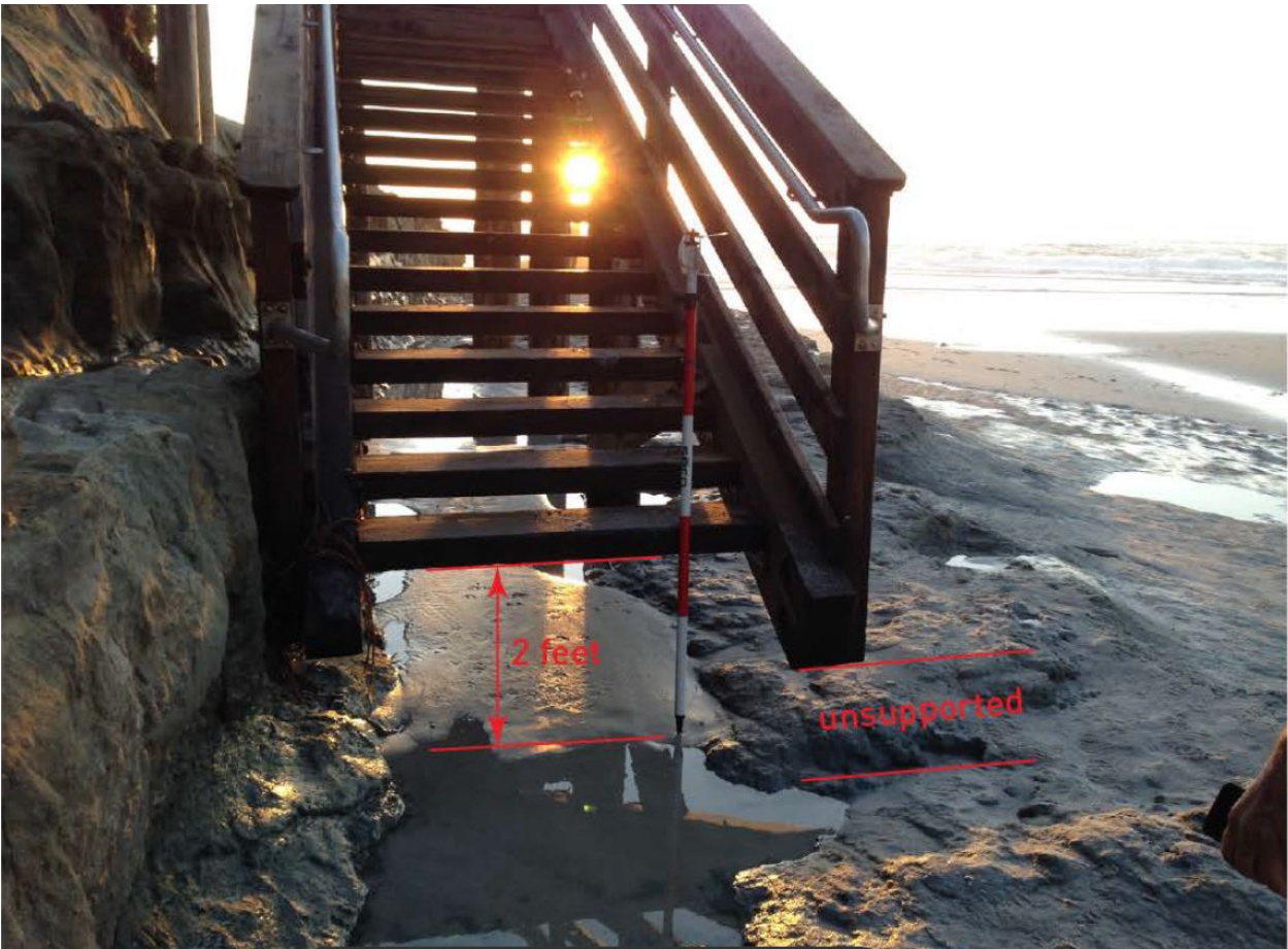
Photograph 39: Undermined Stairway ST4 in February 2016 (Easton Geology)
