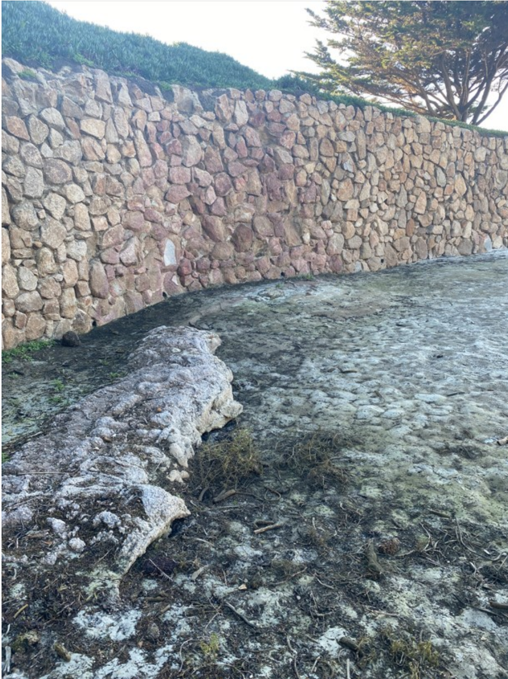
Photograph 23: Concrete Debris on Beach at Base of Seawall S3 on December 22, 2022
