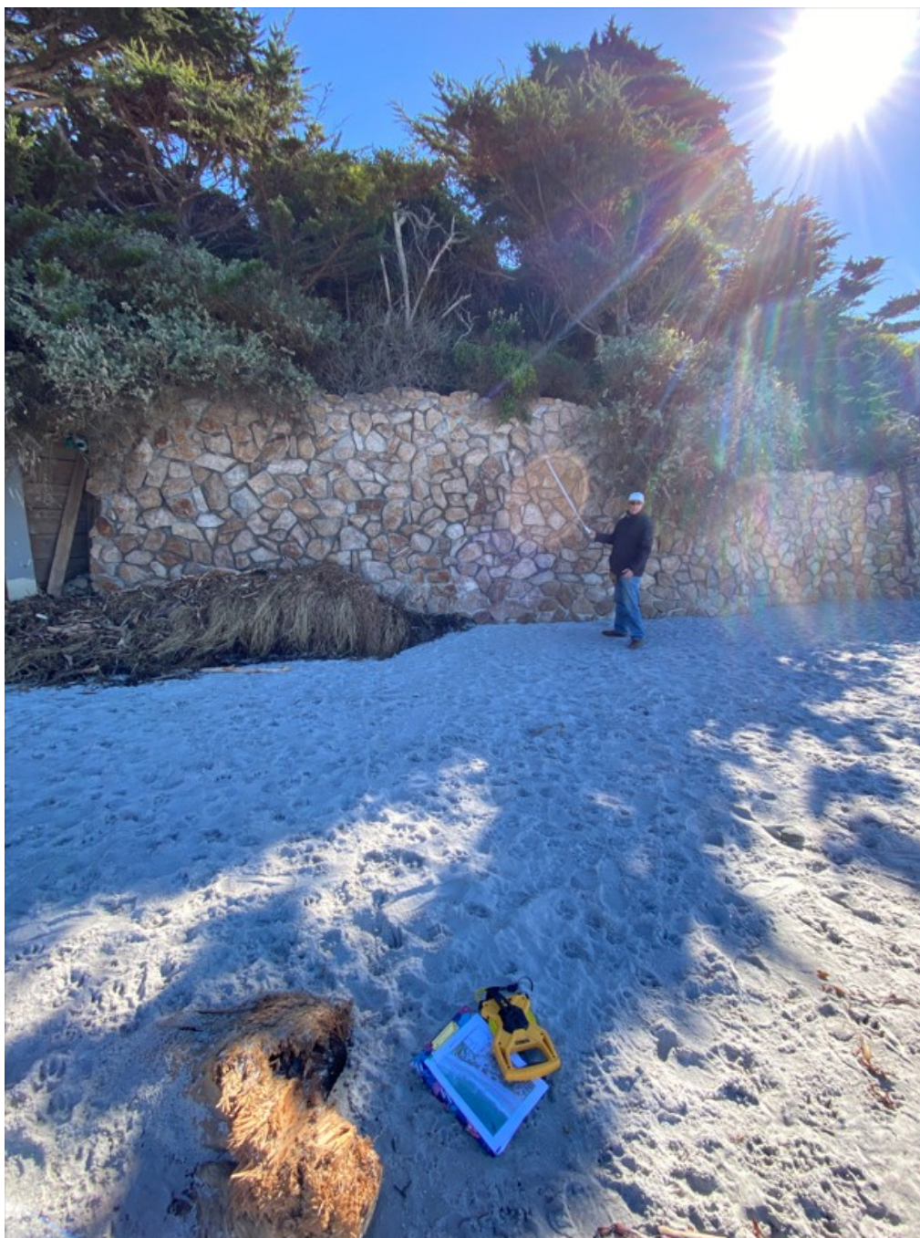
Photograph 73: North Portion of Privately Owned Seawall S11 on January 30, 2023
