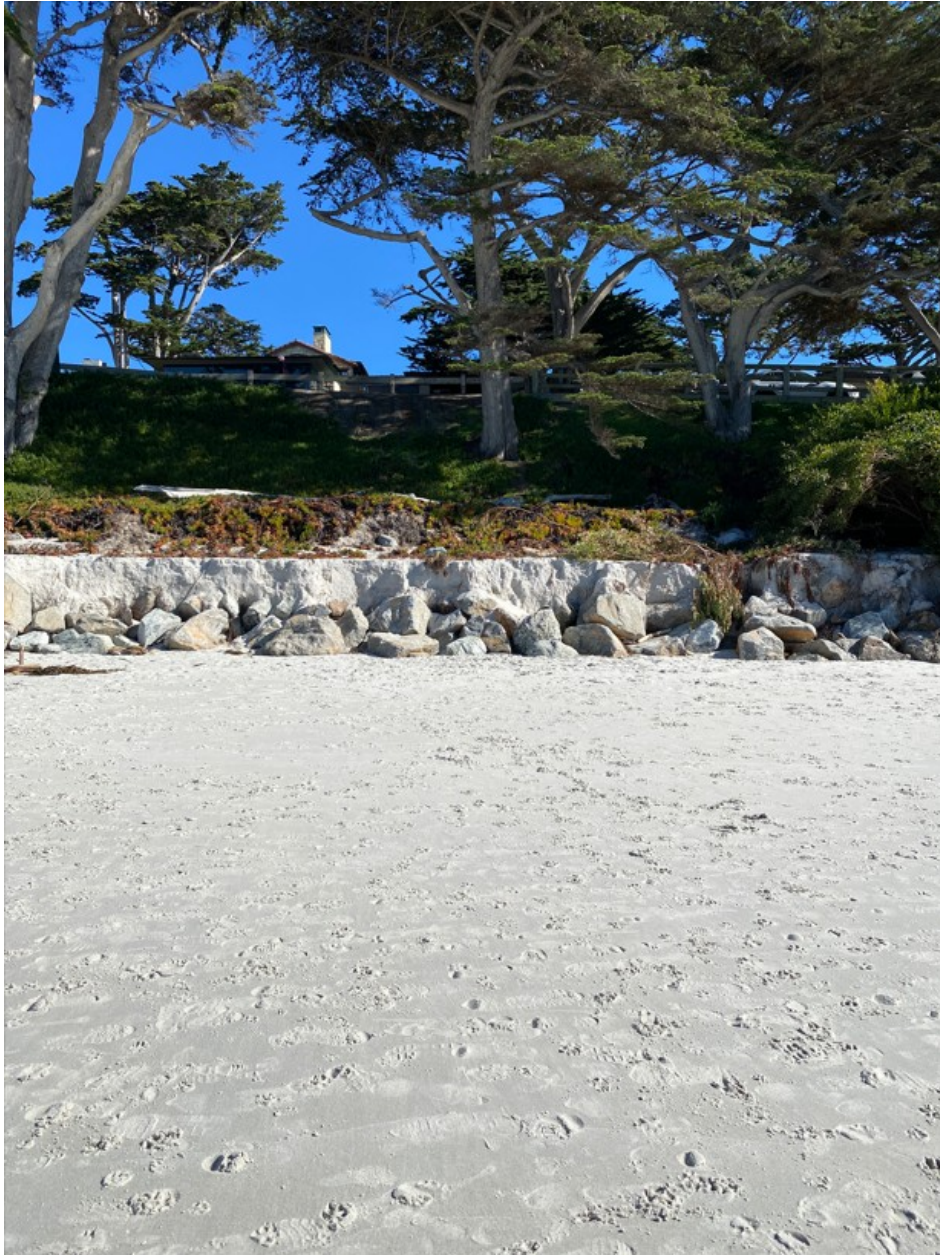
Photograph 77: Southern Portion of Revetment R5 on January 30, 2023 Showing Steep Slope
