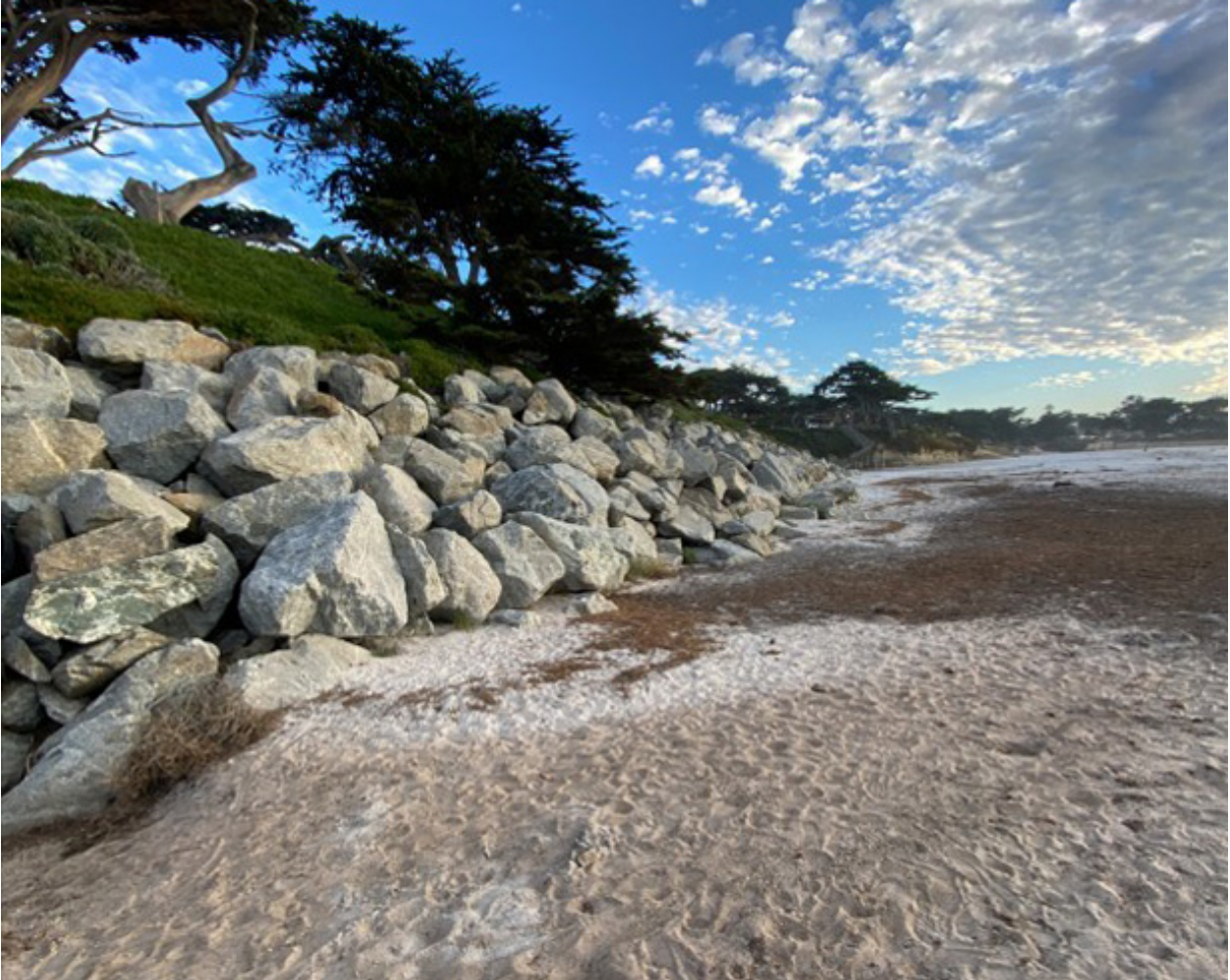
Photograph 54: Over-steepened portion of Revetment R3 on December 22, 2022
