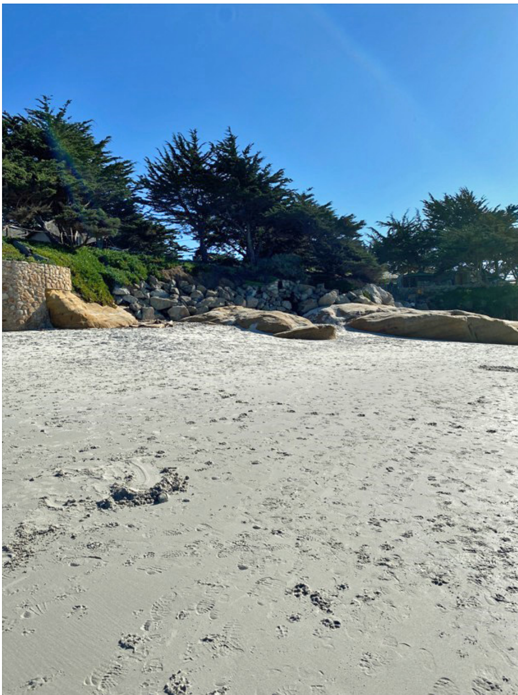
Photograph 20: Showing Revetment R1 and the Southern End of Seawall S3 on January 30, 2023
