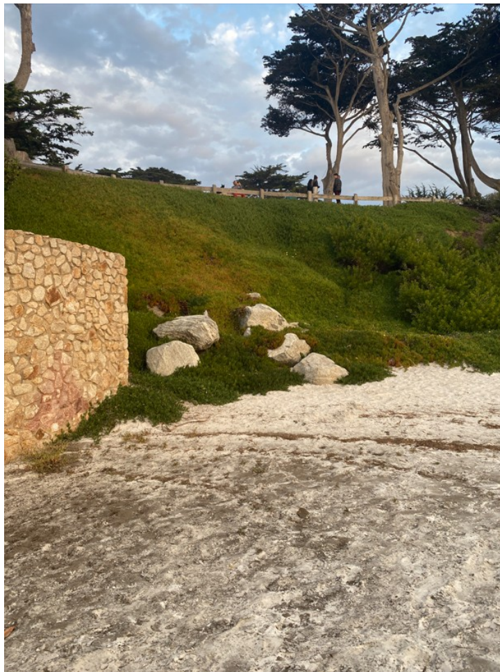
Photograph 63: Showing Few Boulders Exposed at the North End of Revetment R4 On December 22, 2022
