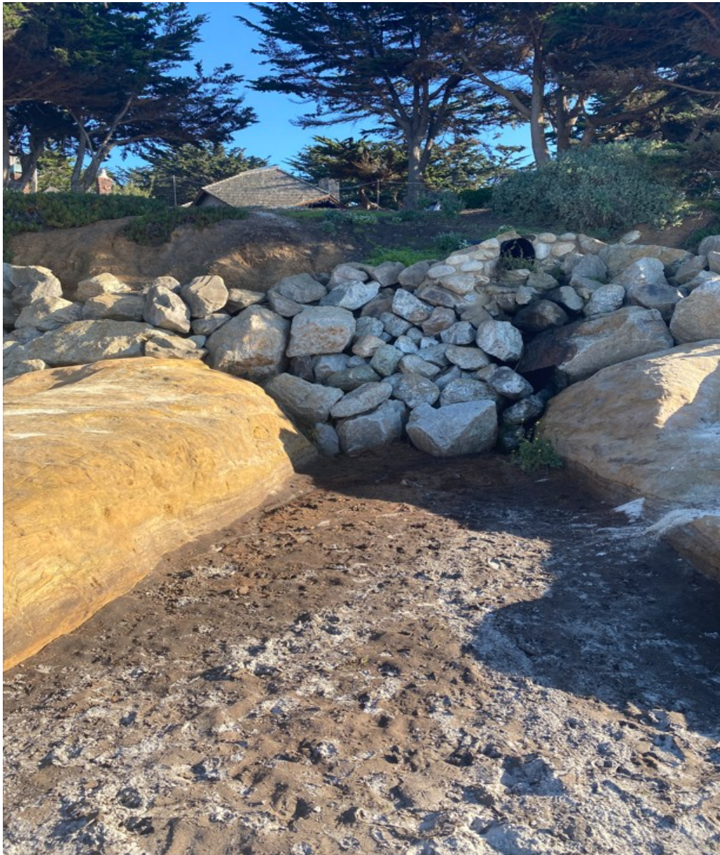
Photograph 18: Revetment R1 Showing Undersized Overly Steep Riprap on December 22, 2022
