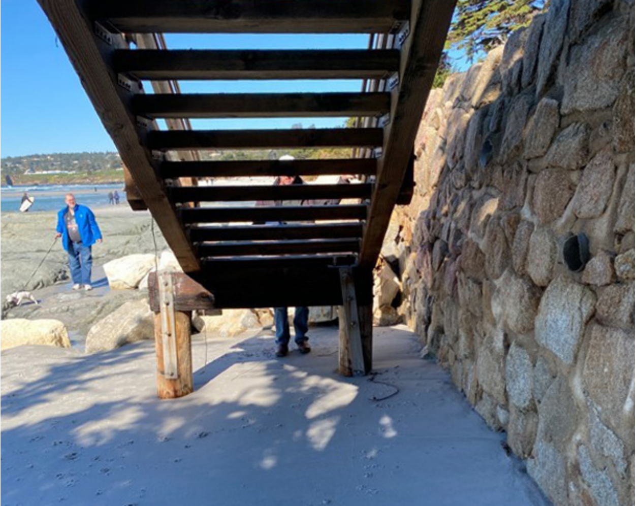
Photograph 74: Stairway ST7 on January 30, 2023 Showing Undermining
