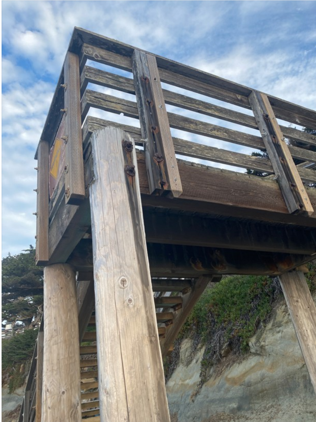
Photograph 41: Showing Corroded Hardware and Split Timbers on Stairway ST4 on December 22, 2022
