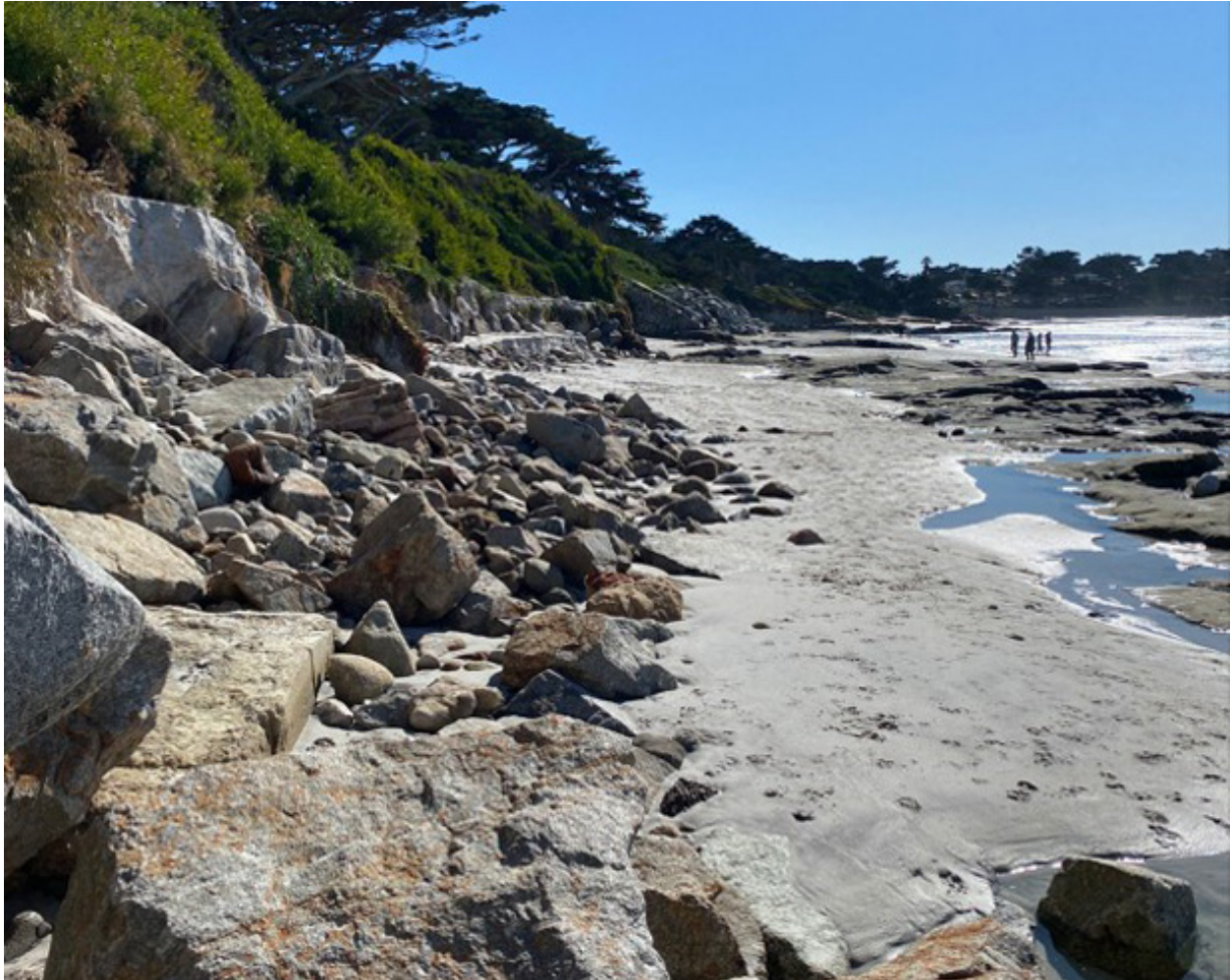
Photograph 61: Northern 1/3 of Revetment R4 Showing Scattered Undersize Riprap Boulders on January 30, 2023
