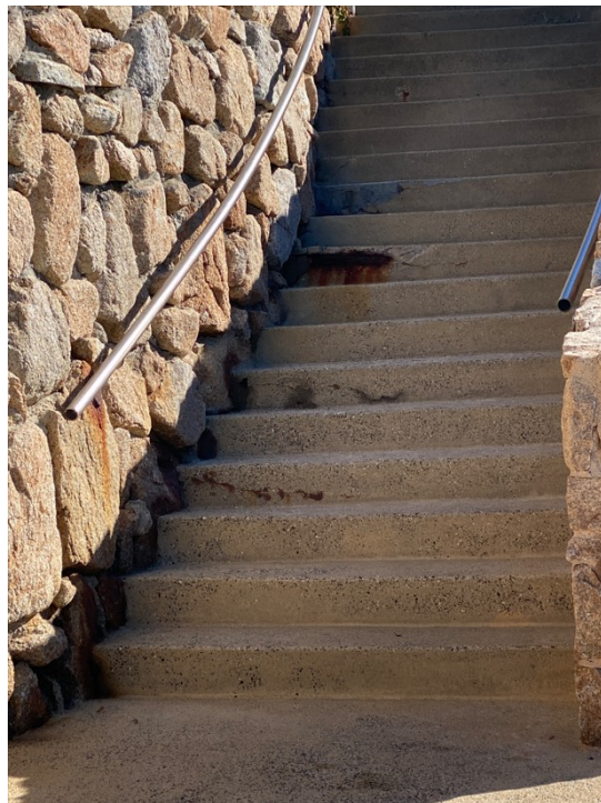
Photograph 67: Stairway ST6 with Tread Deterioration on January 30, 2023
