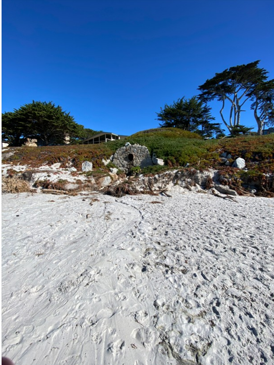
Photograph 89: Revetment R5 and Seawall S9, Showing Small Amount of Riprap Boulders on January 30, 2023
