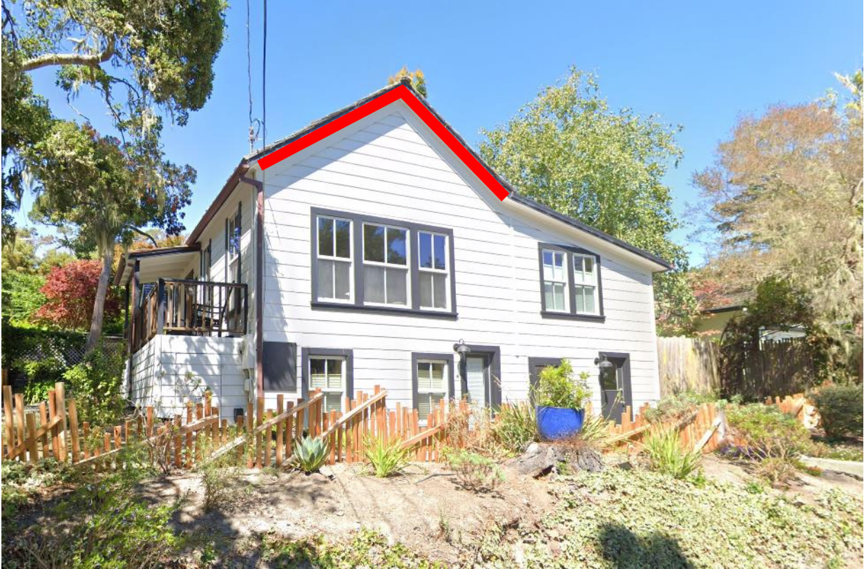
View from 1 st looking northeast. Note: only the pitched gable portion of the roof (highlighted) is proposed to be a metal standing seam roof.
