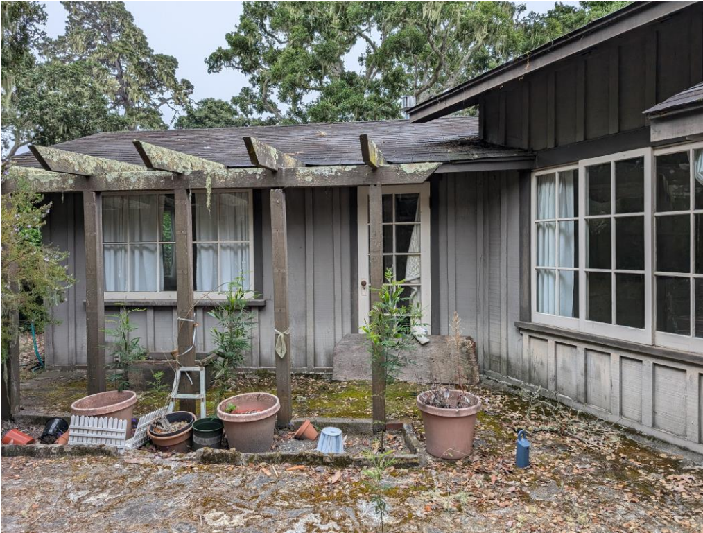
South wing, looking south. Window at image left are fixed, whereas window at image right is a tripartite sliders.
