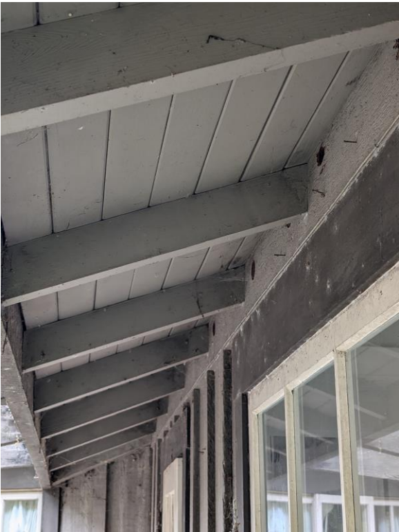
Detail photo of exposed rafters typical of the north and south wings.
