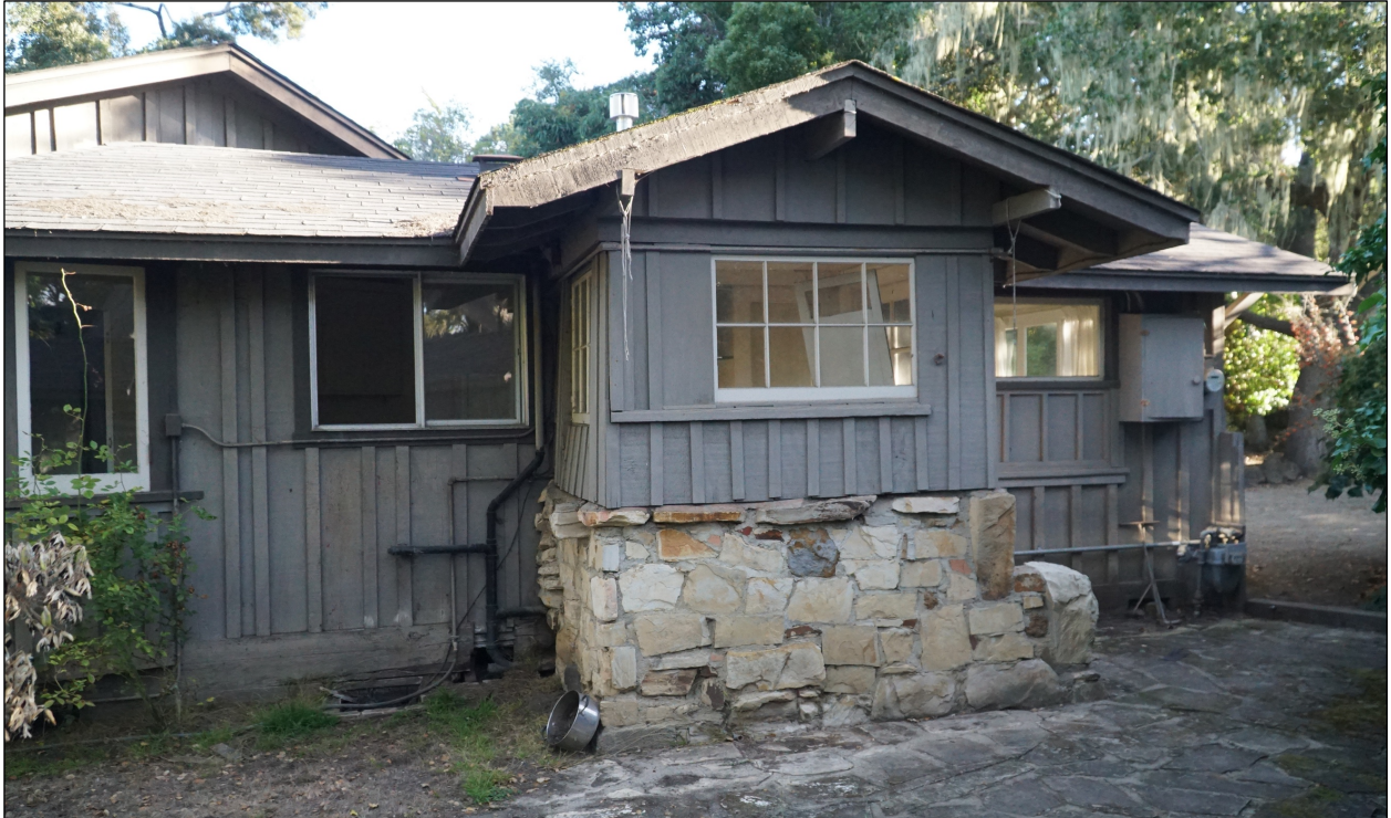
Figure 3. Looking north at a section of south side. The window above the rubblework is clearly not original, nor is the aluminum sliding-sash window is to the left of it.
