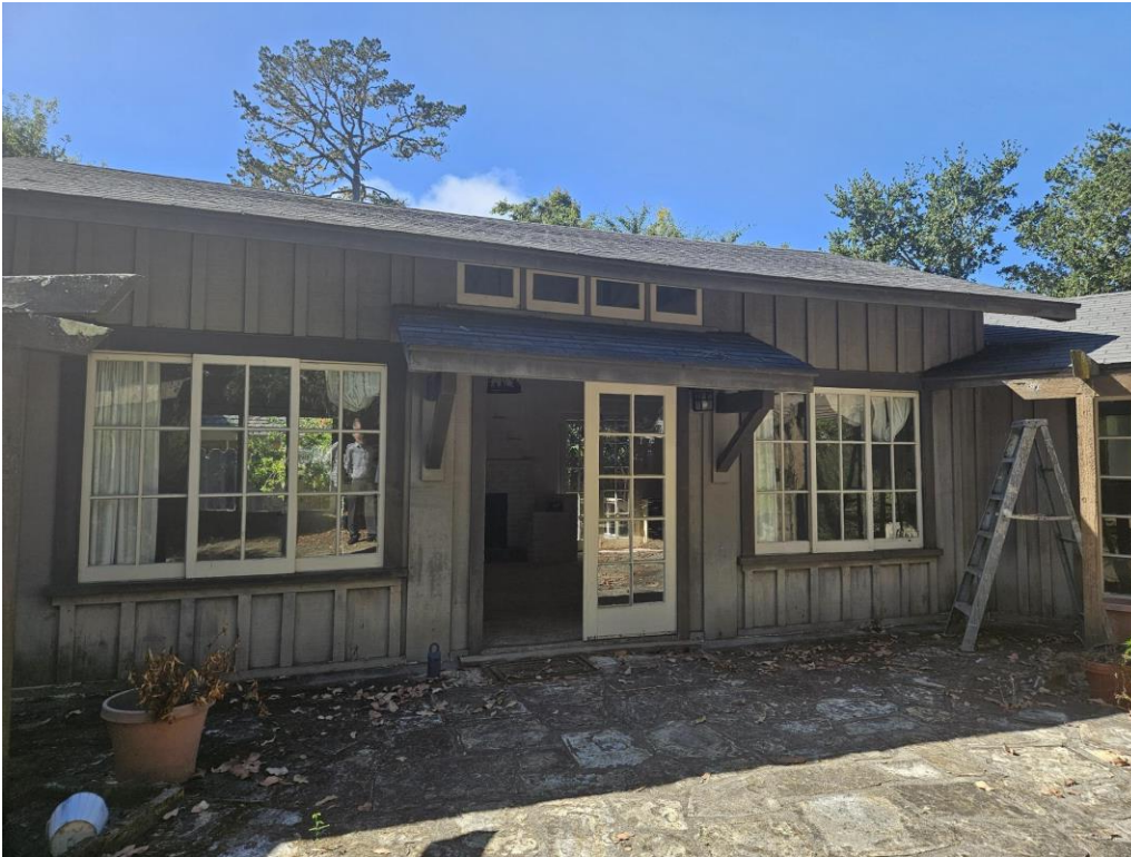
Figure 2: Front entrance with clerestory windows, French doors, and multi-paned wood sliding windows
