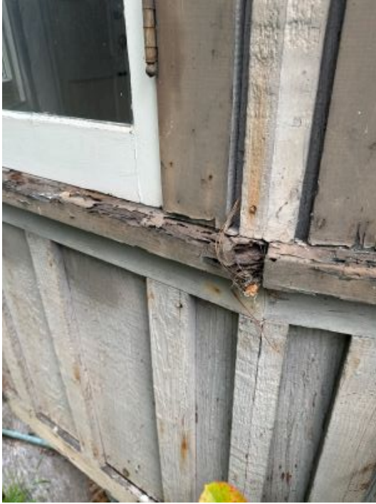
Figure 21 Termite damage at window sill
