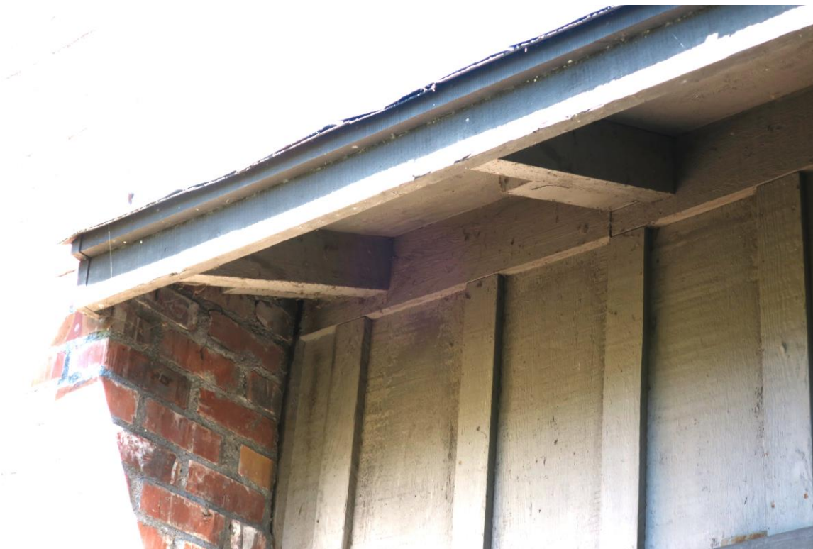
Detail of exposed rafters in the central volume. Note that the exposed rafter tails are truncated and have sistered extensions; this may reflect a construction error where the rafters used were simply not long enough to reach the fascia.
