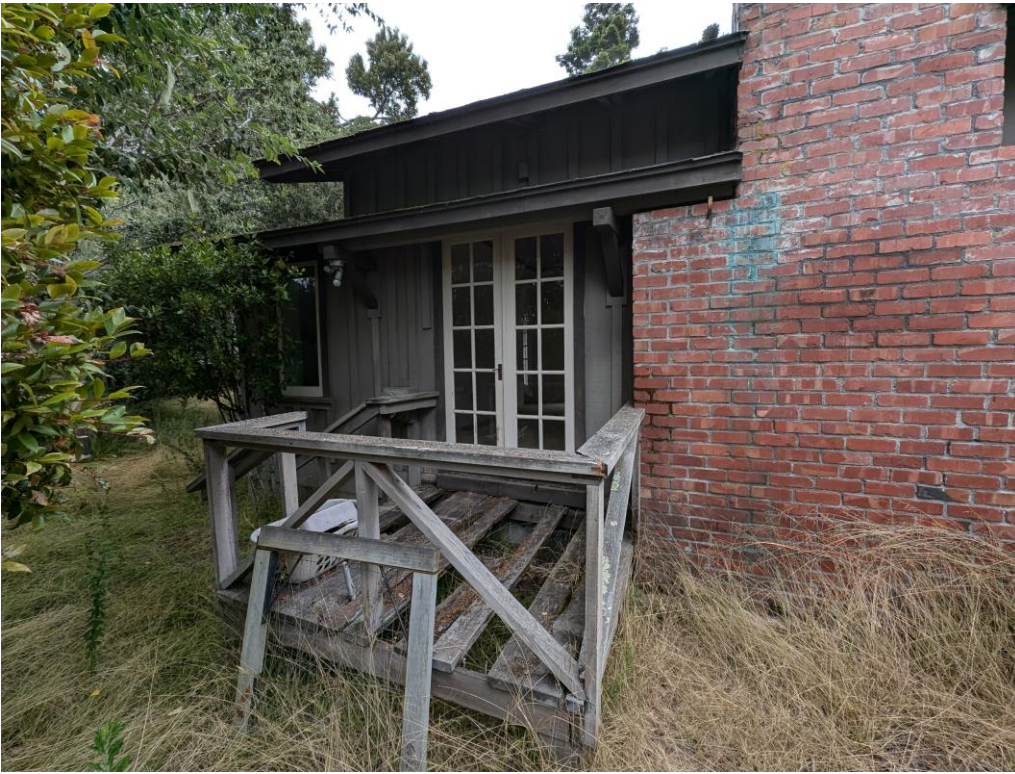
Rear (west) elevation with French doors and exterior brick chimney. Note the narrow shed roof supported by brackets, matching the design of the front entry doors.
