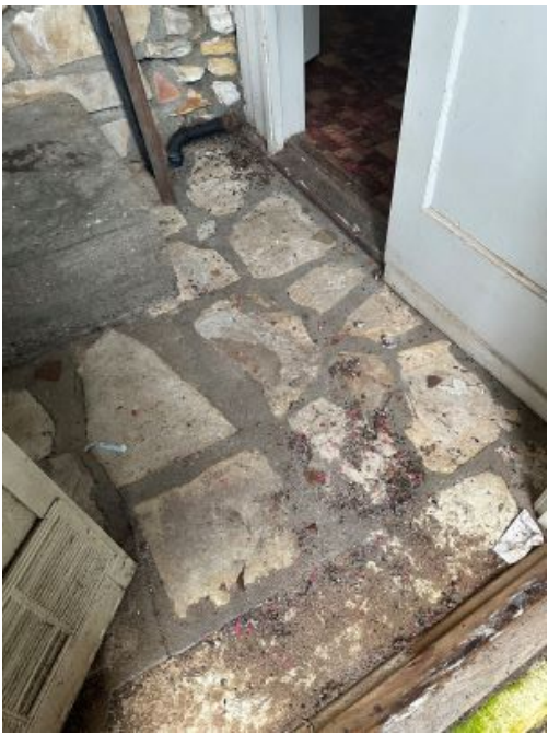
Figure 24 Masonry floor touching wood elements
