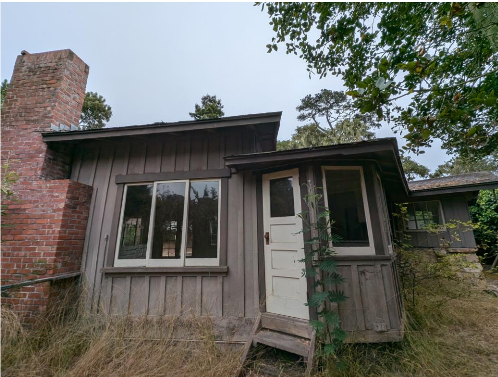
Rear (west) elevation, with exterior brick chimney at image left, pentagonal bay with casements at image center, and service porch image right.
