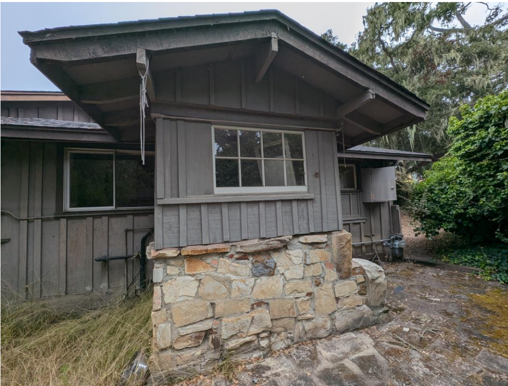
South wing service porch, looking northeast. Aluminum window at image left, and what appears to be a non-original or altered window opening in the foreground.
