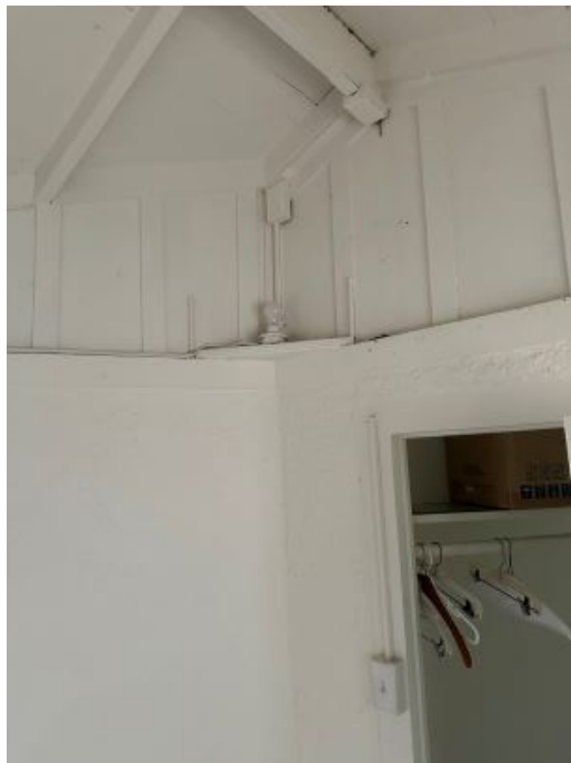
Figure 16 Stucco on interior walls and exposed wiring
