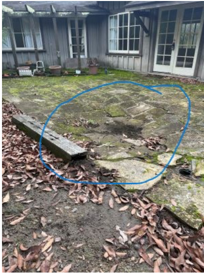
Figure 1 Area of patio subsidence
