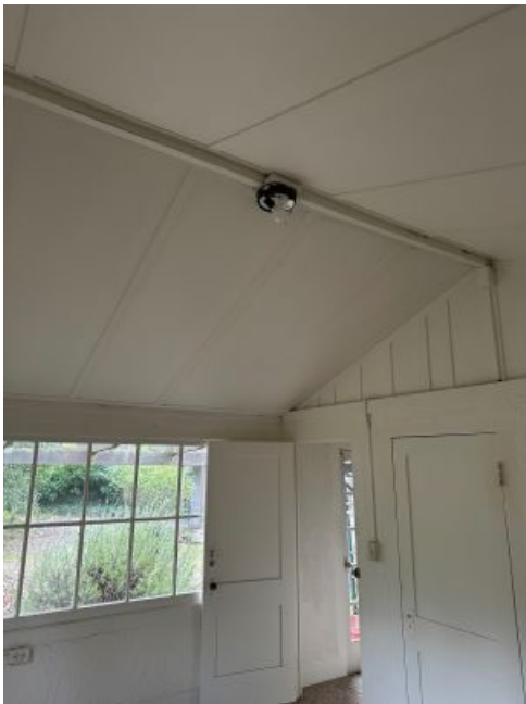
Figure 8 Bedroom ceiling with 2x6 ridge board and wood fiber insulation finish material
