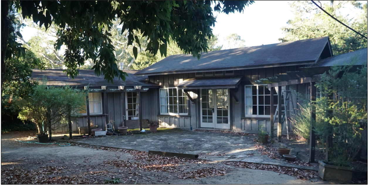
Figure 1. Looking west at east side and adjoining wings. The presence of subsurface water carrying soil away is evident at the front of the patio, directly below the two French doors.
