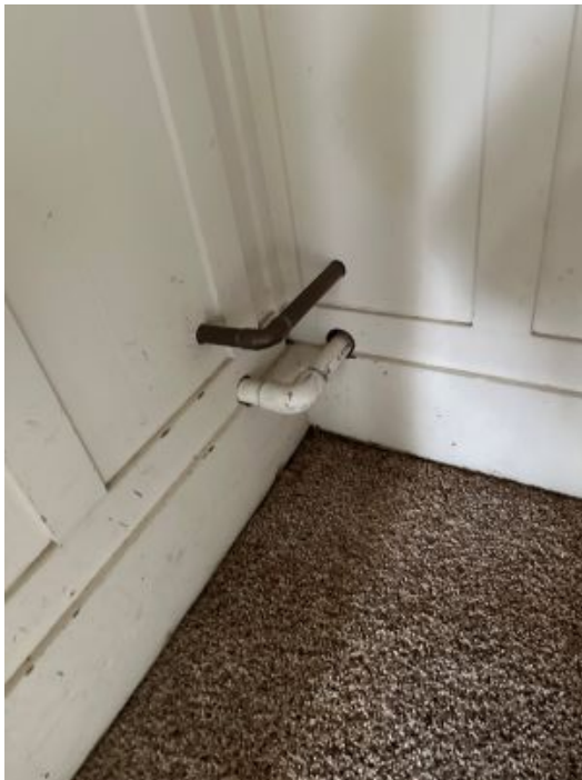
Figure 14 Surface run plumbing in bedroom
