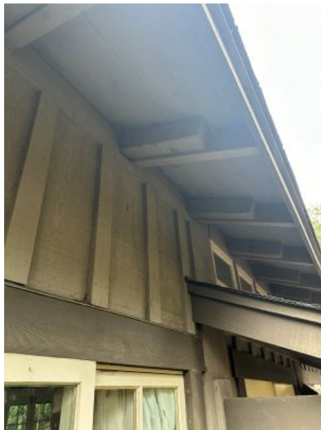
Figure 6 Structural rafters too short
