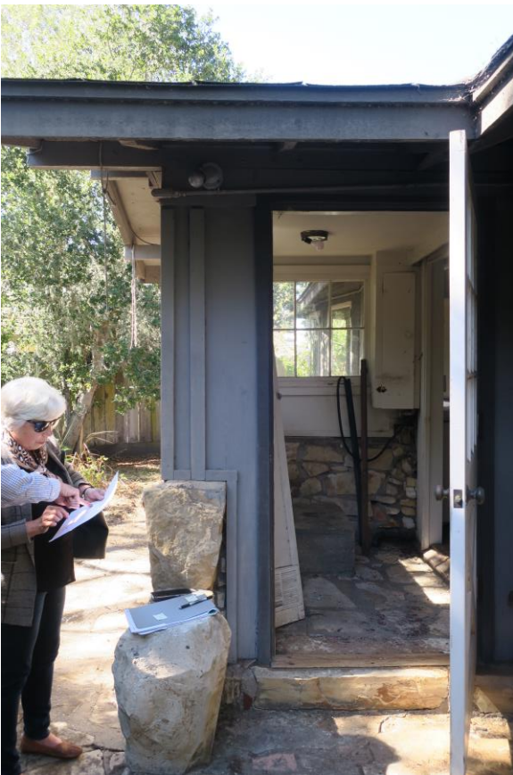
Service porch, with rubble stone base and what appear to be non-original window openings.
