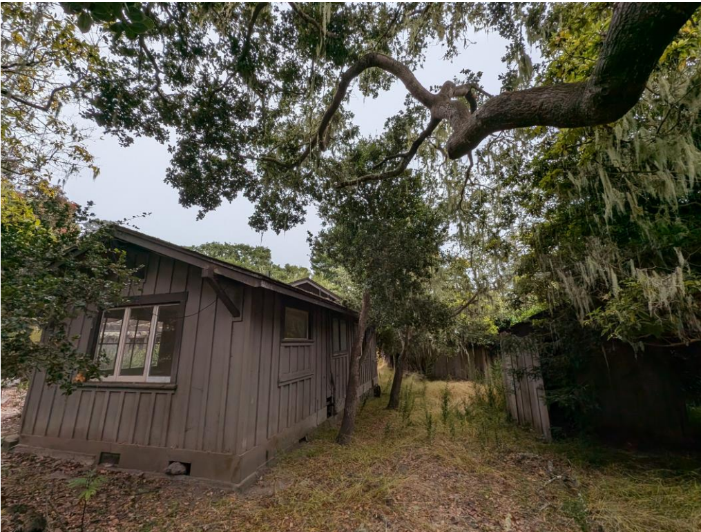
North wing, looking west. Note tripartite slider in the gable end, and the partially infilled window opening on the north elevation. Note detached garage at image left.
