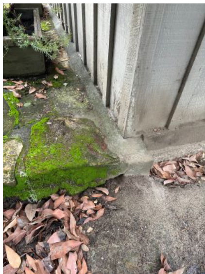
Figure 2 Patio contacting wood siding
