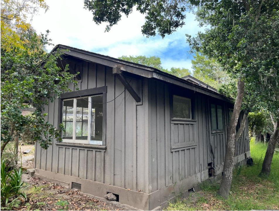
Photograph 3: Northeast (end) and northwest (rear) elevations showing single-light sliding wood windows, partially enclosed window openings, and aluminum sliding-sash, camera facing southwest.
