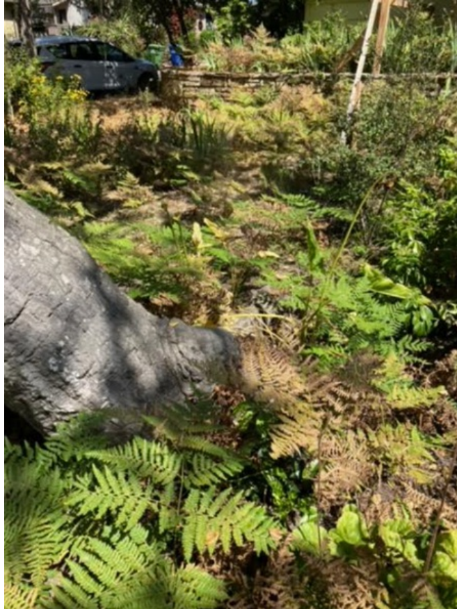
Figure 5. Trunk of tree located nearest to encroaching retaining wall. Subject tree roots (partially visible through foliage) are directed toward interior of site away from retaining wall.
