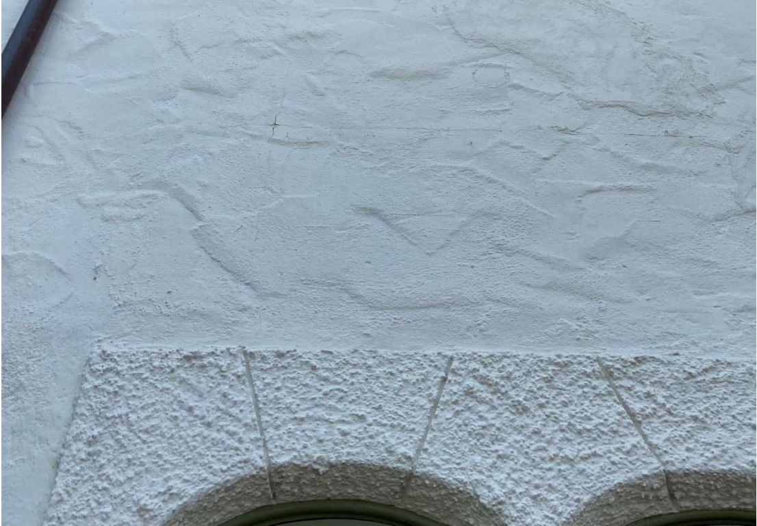
Photo #7, hairline cracking in plaster above double windows by main entry
