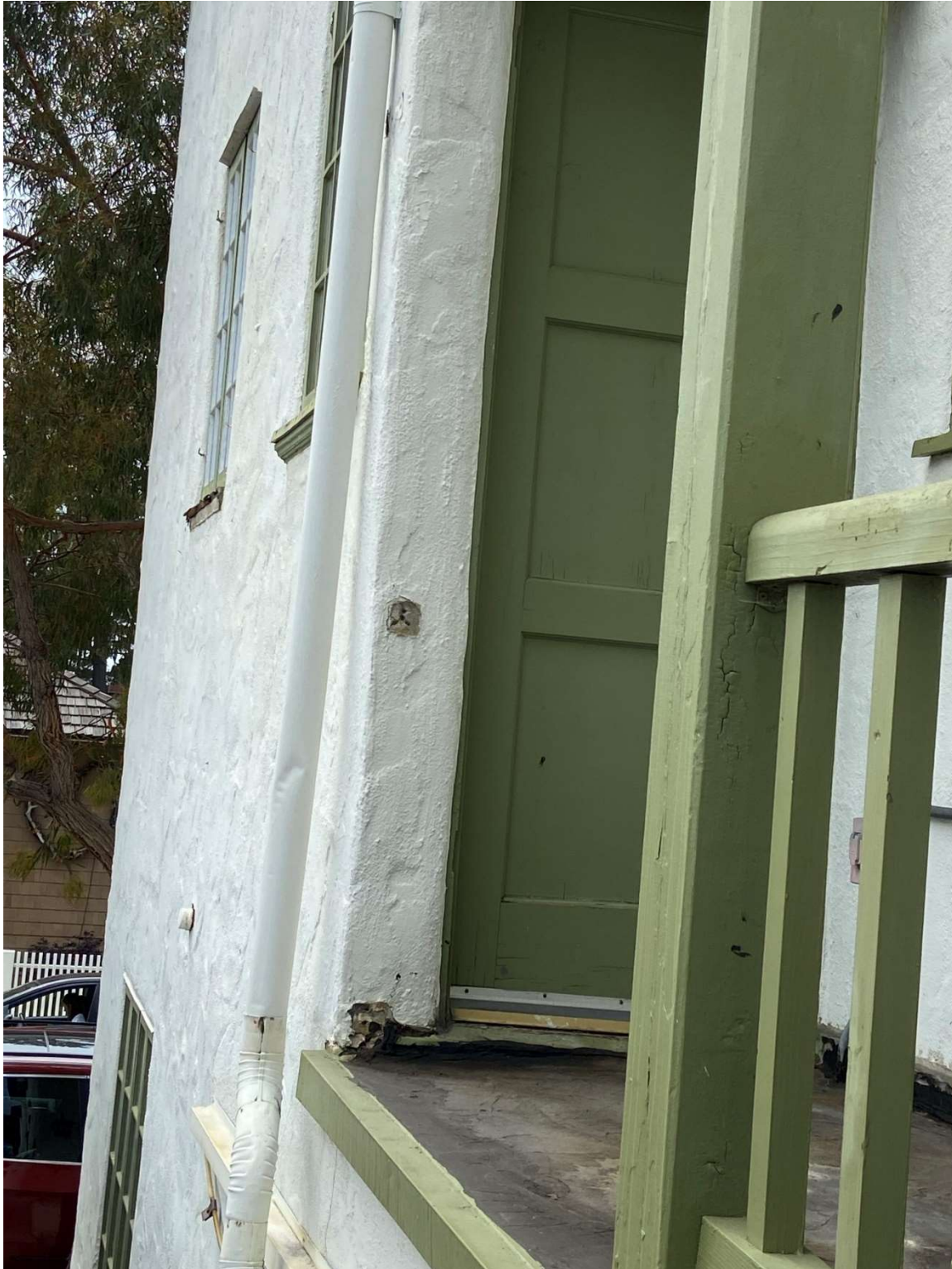
Photo 14, Water damage at upper-level balcony
