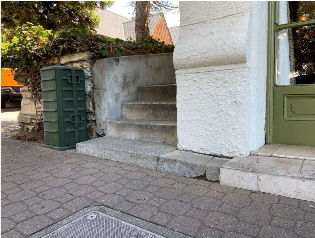
Photo #10, cracked step/foundation at Northwest building corner
