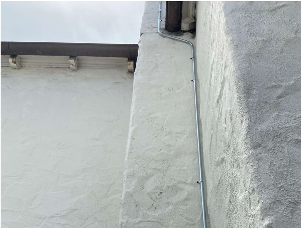
Photo #11, damaged rafter tails at roof as seen from courtyard
