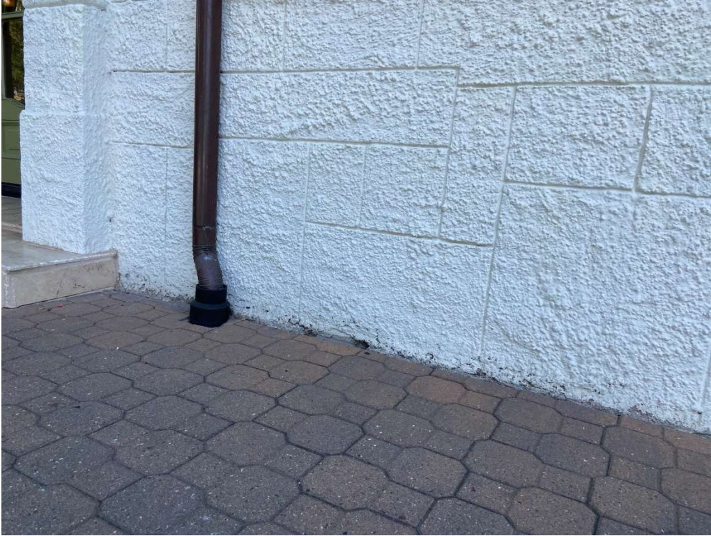
Photo #9, holes in foundation near Northwest building corner
