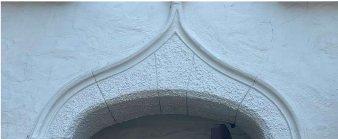
Photo #8, radial cracking in plaster above main entry doors.
