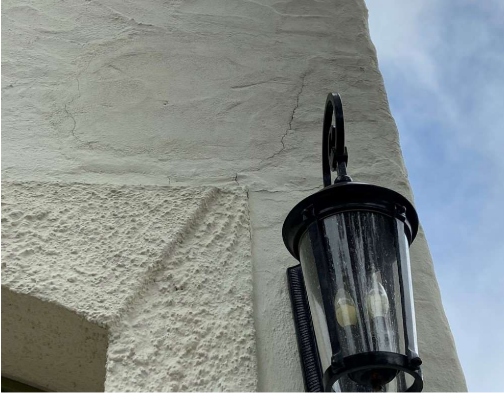
Photo #5, radial plaster cracking at Southwest building corner
