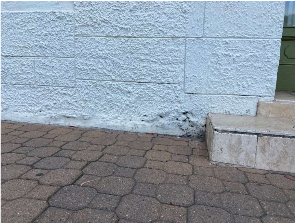
Photo #6, holes in foundation, plaster and tile at Southwest corner
