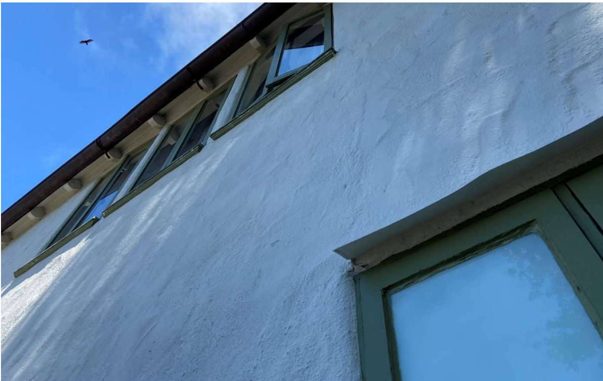
Photo #12, bent/damaged flashing at second level opening
