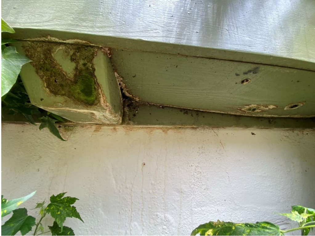
Photo #12, rotted supports at exterior planter box
