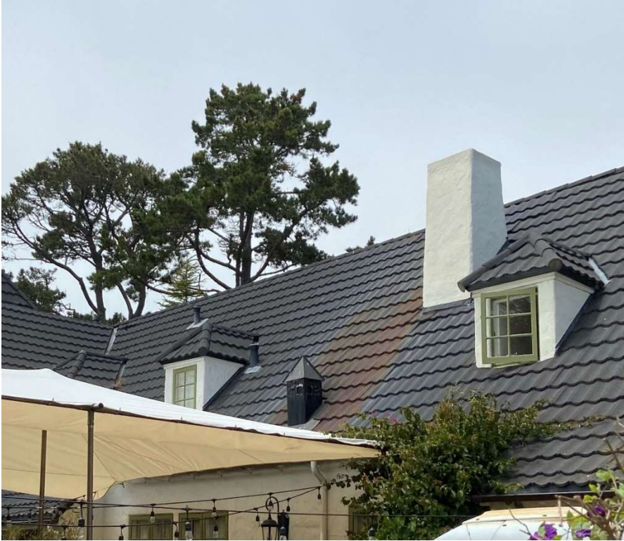
Photo #10, weathered/oxidized roofing at central courtyard
