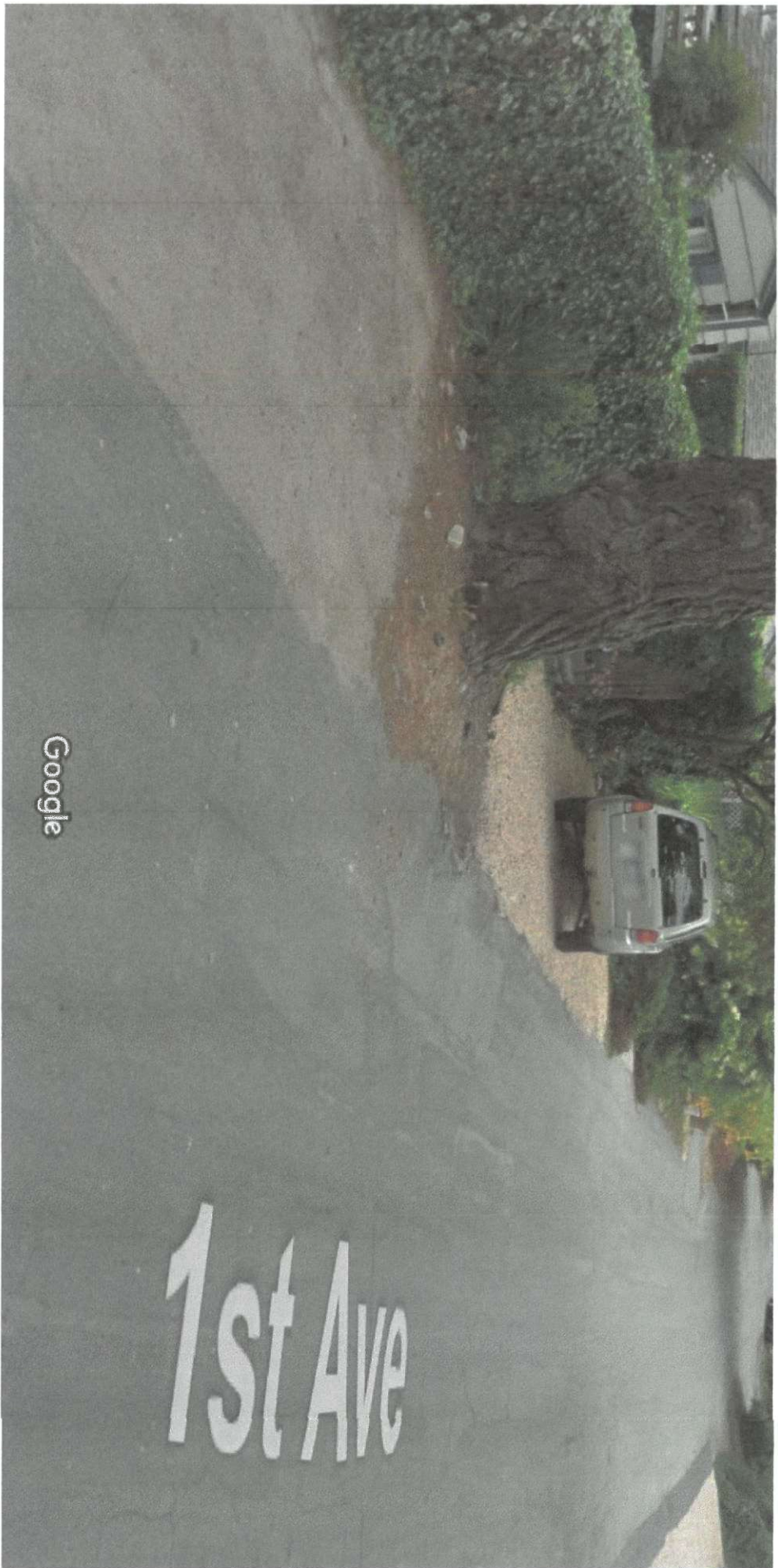
previous root disturbance and repair, prior to 2011
