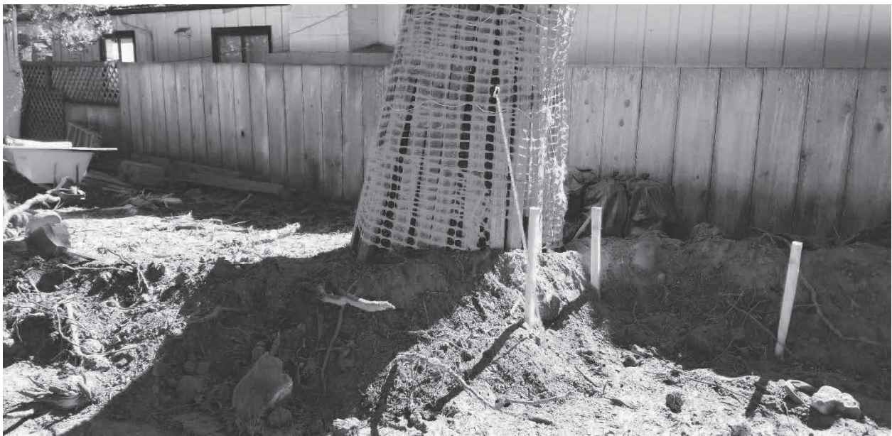
Figure 6: Looking south at Tree #5, Note roots ripped from ground with in 1-foot of trunk.
