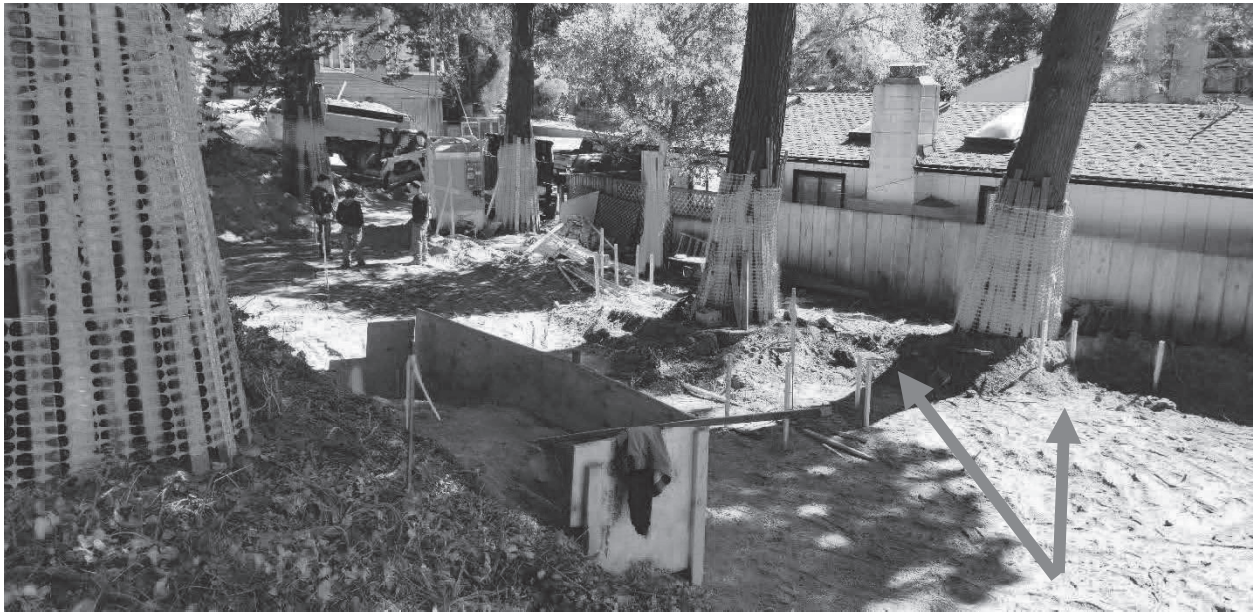
Figure 5: Looking southeast from Tree #7, red arrows note how close excavation was preformed near trees 4 and 5.
