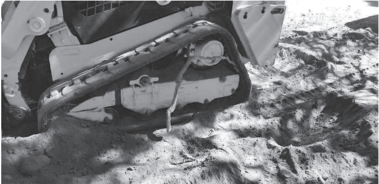
Figure 7: Skid-steer loader operating on site, note roots stuck in tracks an indication that little to no caution of roots was taken during excavation.
