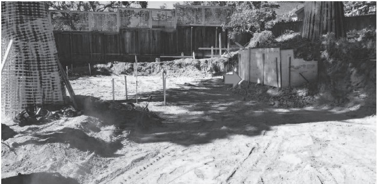
Figure 3: Looking west inside excavation area, red arrow shows box that was constructed around exposed roots of tree #7.
