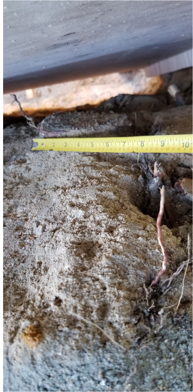
Figure 5: Severed root that measured 6.5-inches in diameter.
