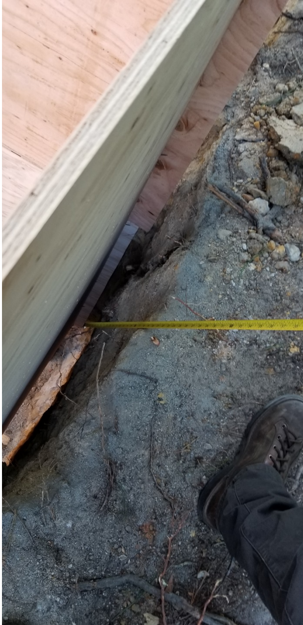
Figure 4: Looking down southern wall of excavated area where severed roots were found.
