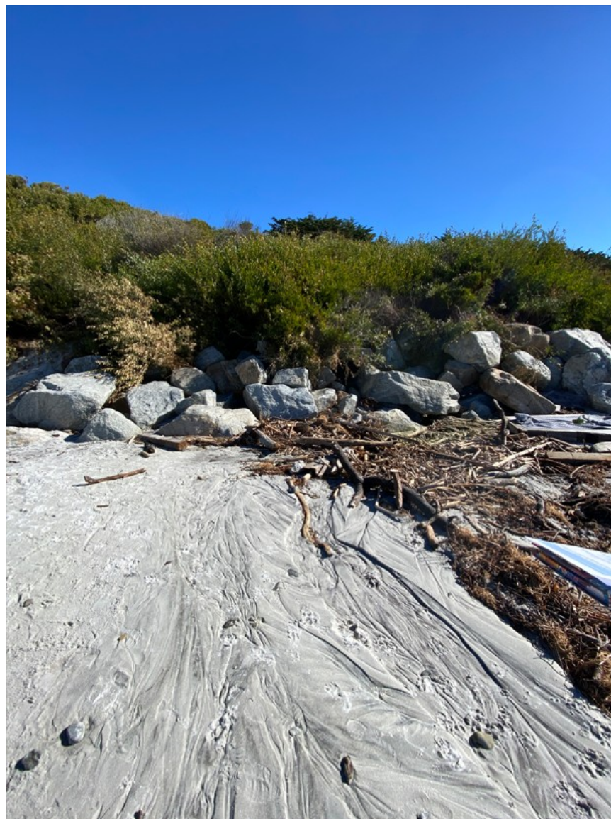
Photograph 91: Revetment R6 Showing Small Amount of Rip-rap Boulders on January 30, 2023
