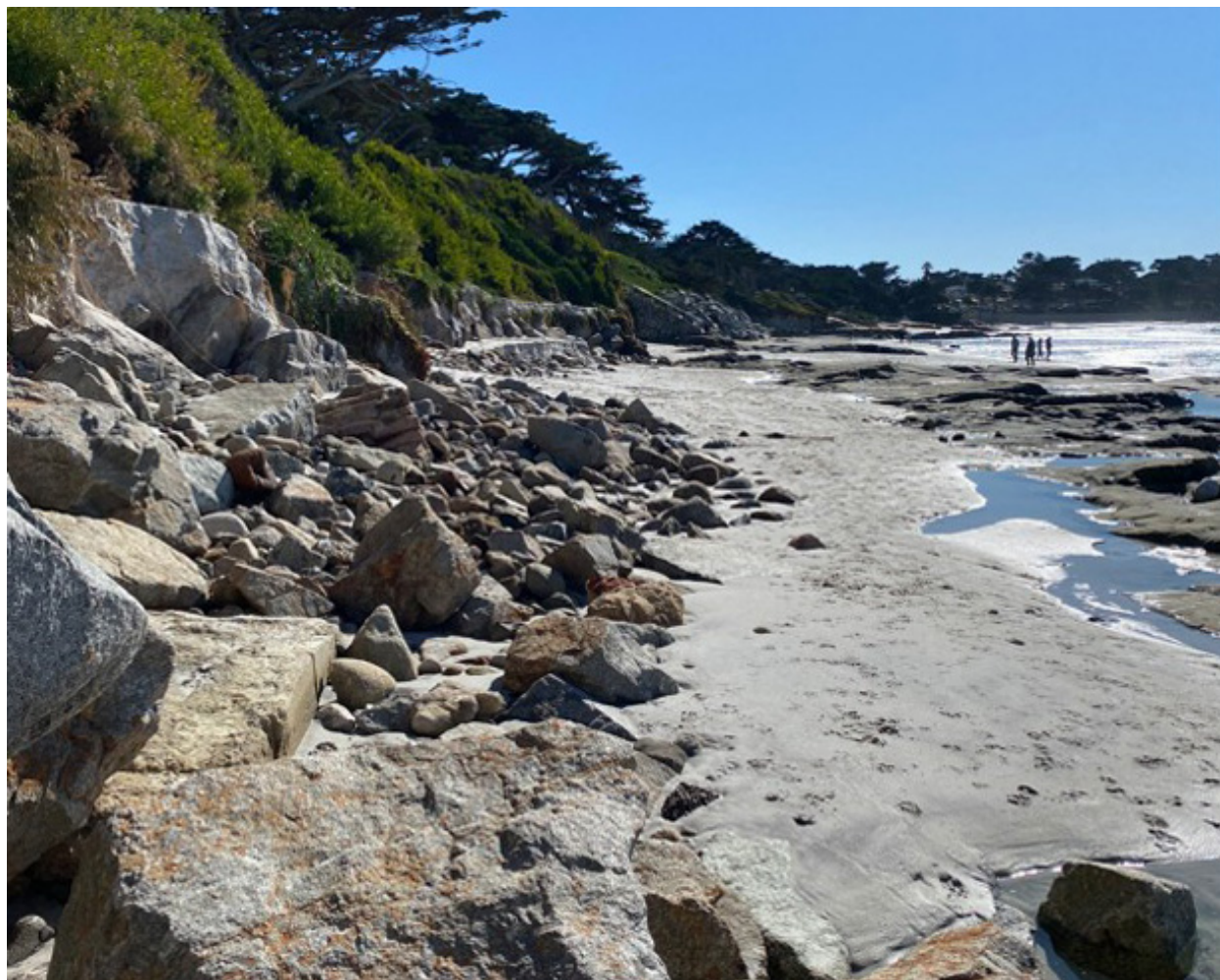
Photograph 61: Northern 1/3 of Revetment R4 Showing Scattered Undersize Riprap Boulders on January 30, 2023
