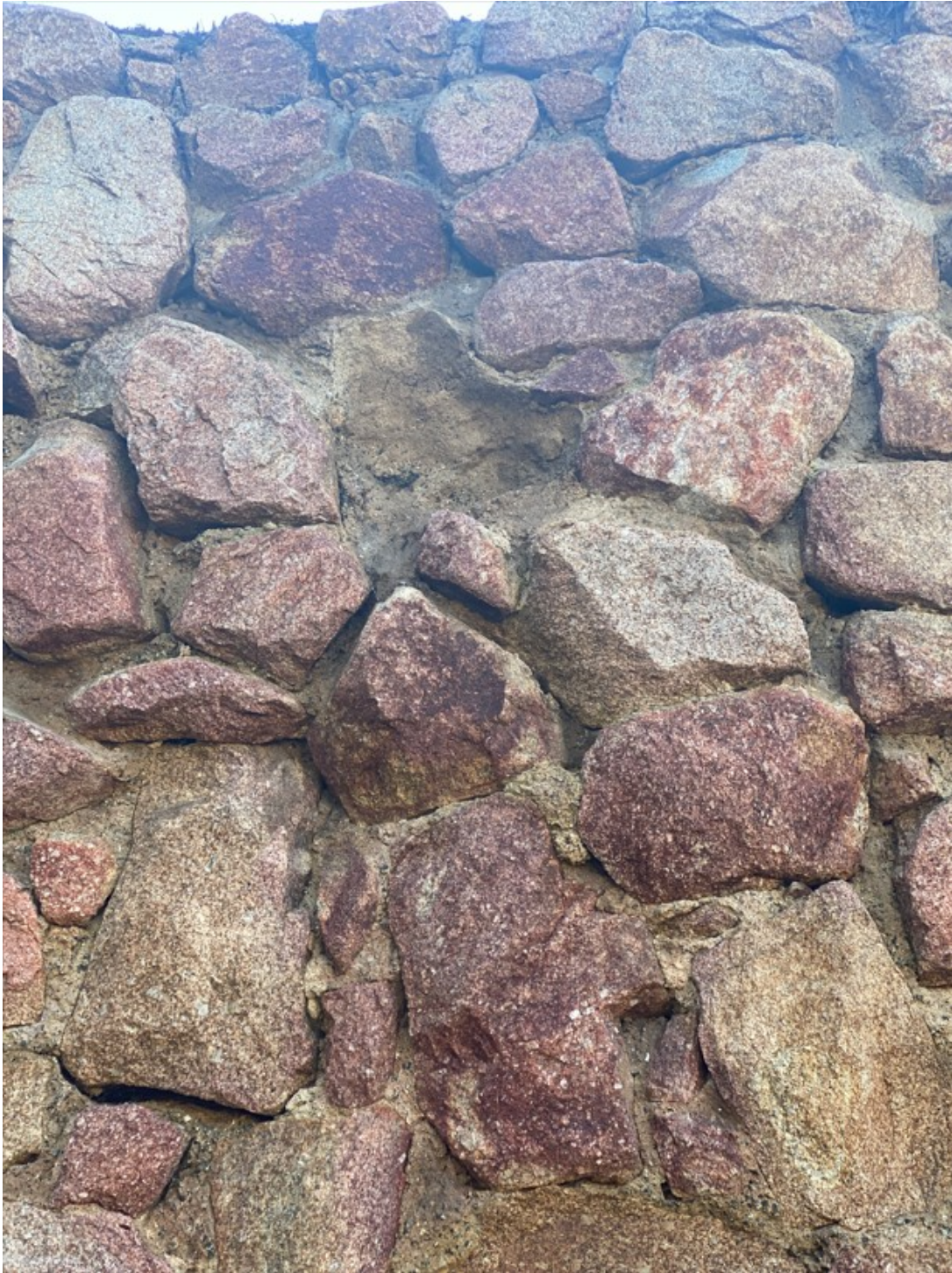
Photograph 26: Seawall S3 Showing Missing Rock on December 22, 2022
