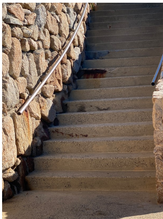
Photograph 67: Stairway ST6 with Tread Deterioration on January 30, 2023
