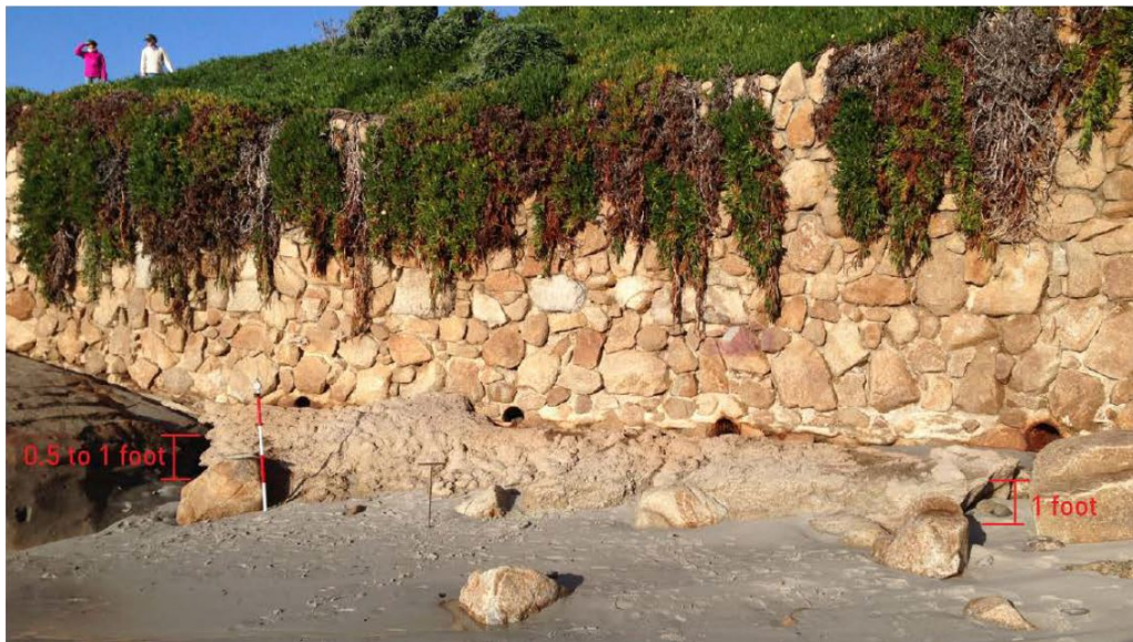
Photograph 24: Southern End of Seawall S3 in February 2016 Photographed by Easton Geology Showing Pumped Concrete Repair of Undermining of Seawall S3
