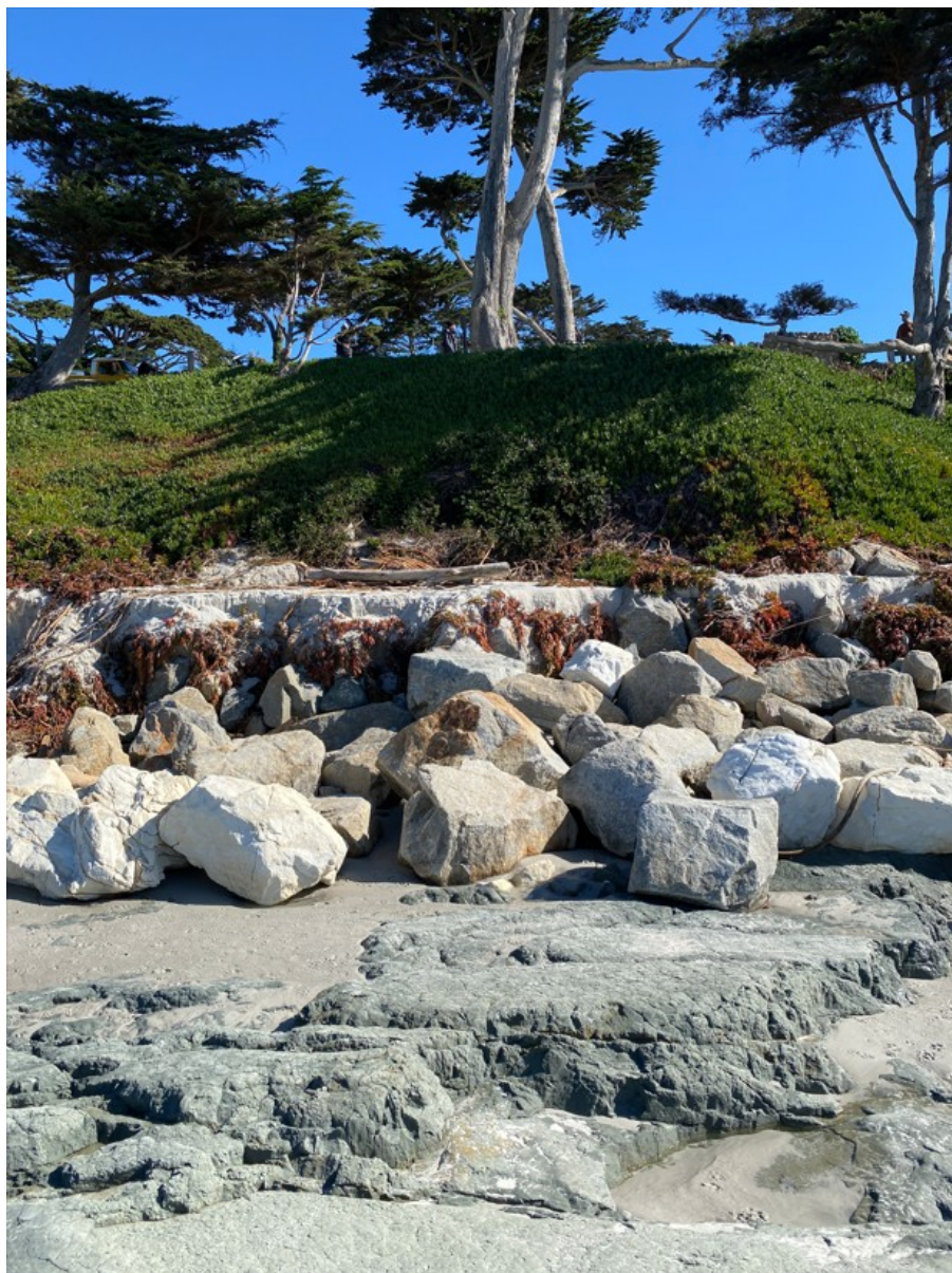
Photograph 75: South Portion of Revetment R5 on January 30, 2023 Showing Bedrock Platform Below Beach Sand and Old Erosional Scarp in Ice Plant Above Revetment
