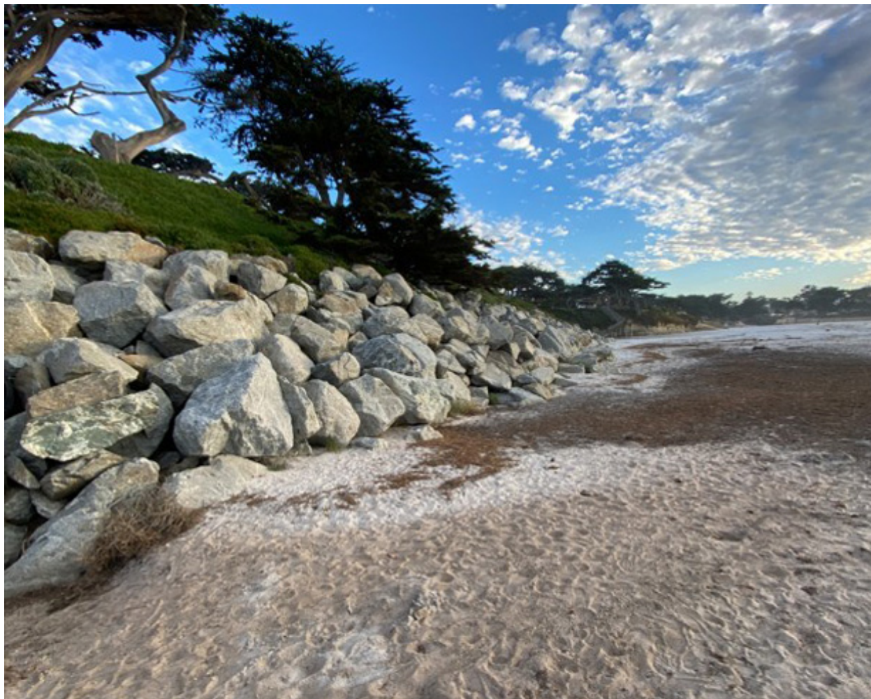
Photograph 54: Over-steepened portion of Revetment R3 on December 22, 2022
