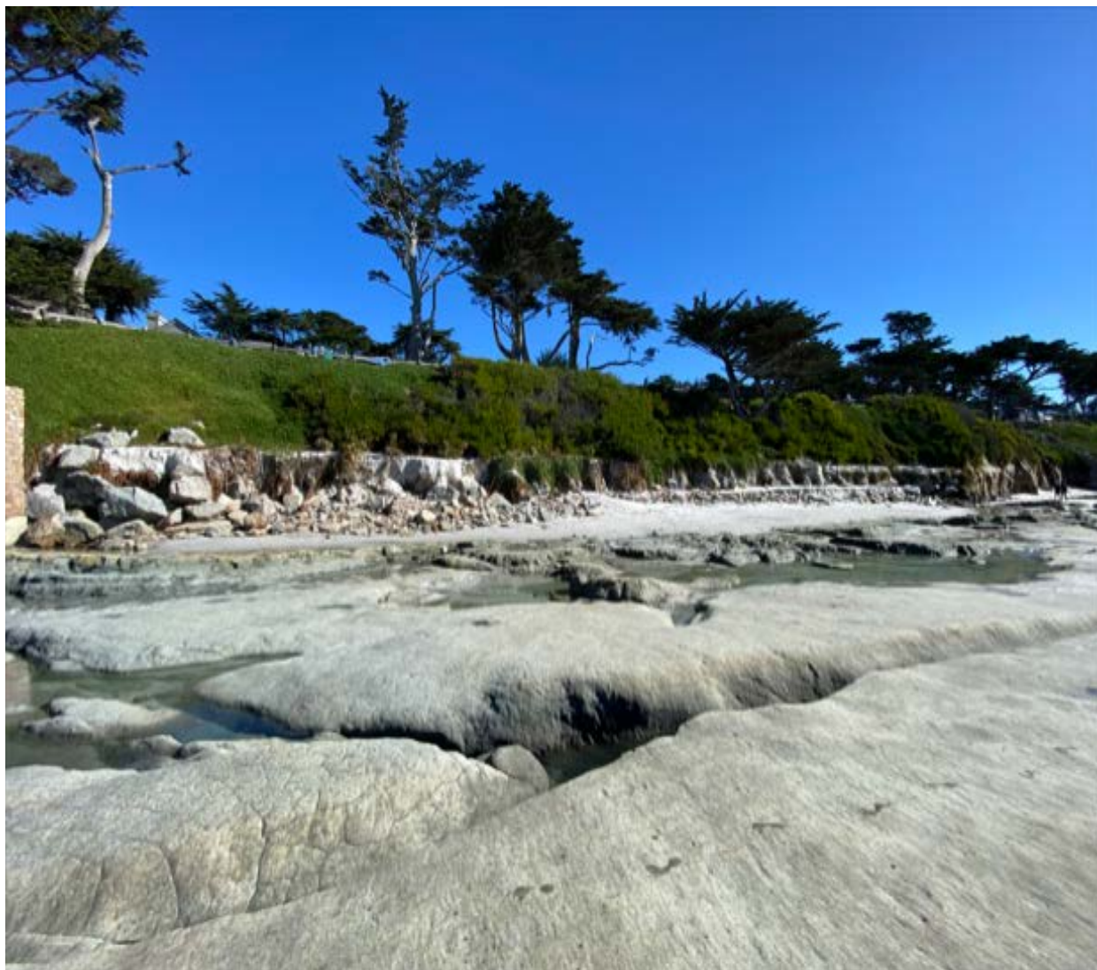
Photograph 62: Northern 1/3 of Revetment R4 Showing Very Undersized Scattered Rock on January 30, 2023
