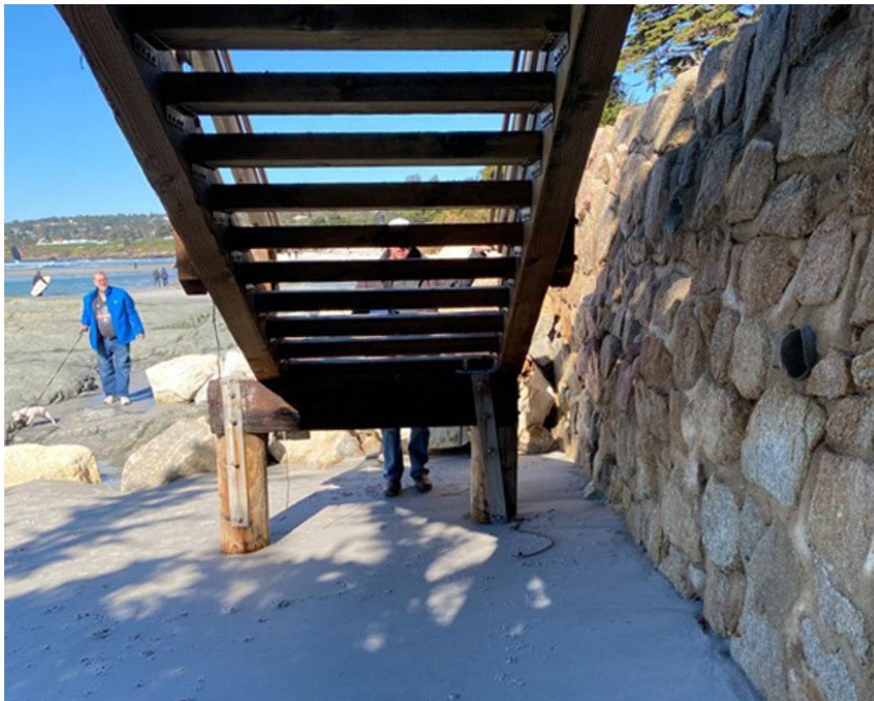
Photograph 74: Stairway ST7 on January 30, 2023 Showing Undermining
