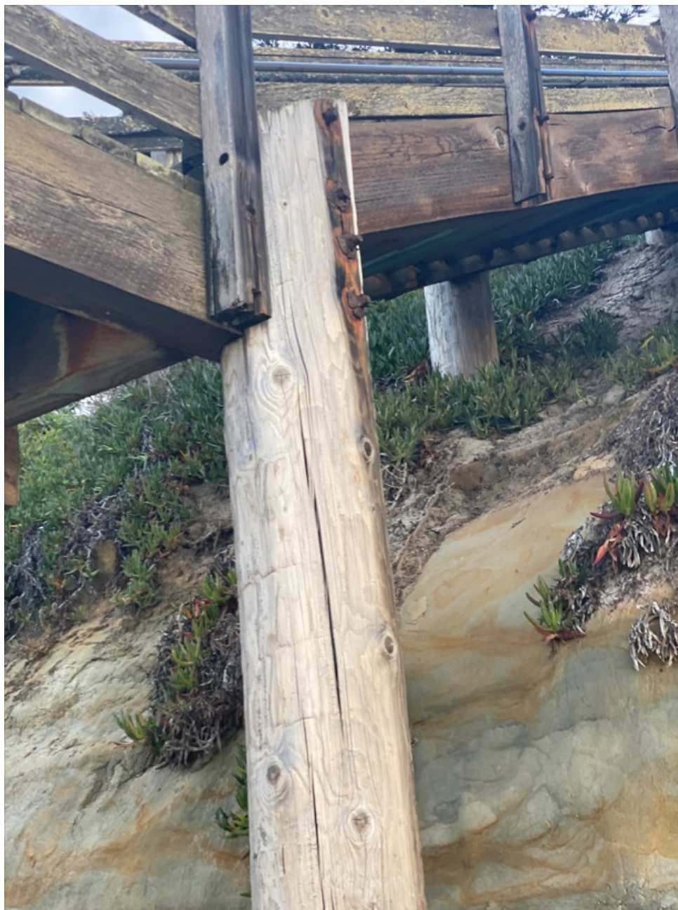
Photograph 42: Showing Corroded Hardware and Split Timbers on Stairway ST4 on December 22, 2022
