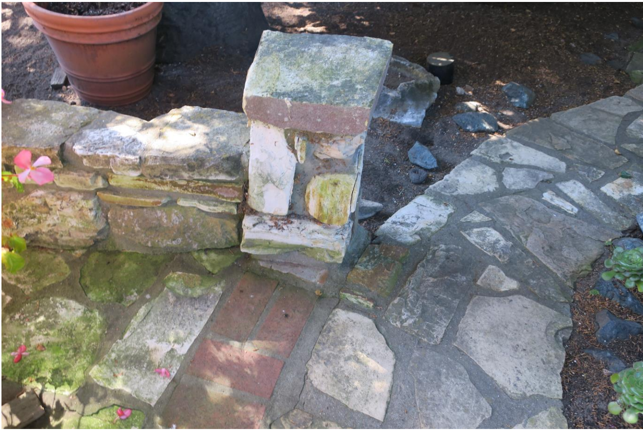
Detail photo of Carmel stone and brick walkway and garden wall in front yard.
