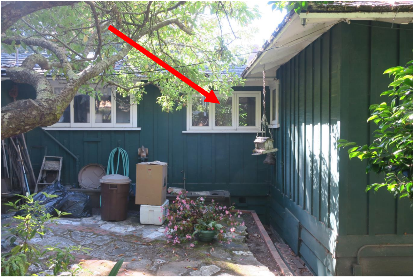
North side elevation, looking south. Arrow indicates non-original window (narrower sill, no extended lintel)
