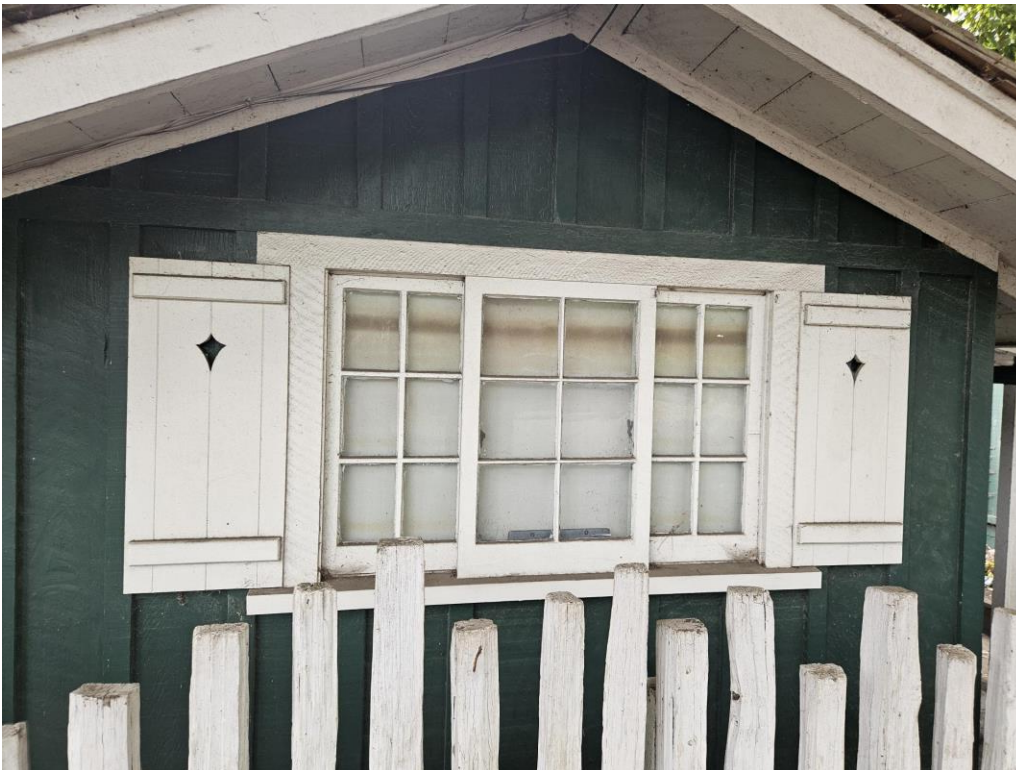
Figure 2: View of sliding wood sash, plank shutters, and extended lintels and sills.
