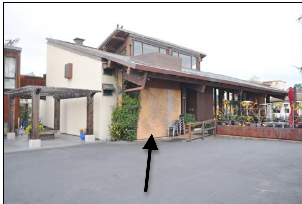
Figure 5. Looking northwest at the east elevation of the Bank Building, the ornamented concrete wall shown.
