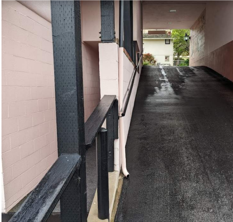
Figure 29 – Downspout onto Driveway
