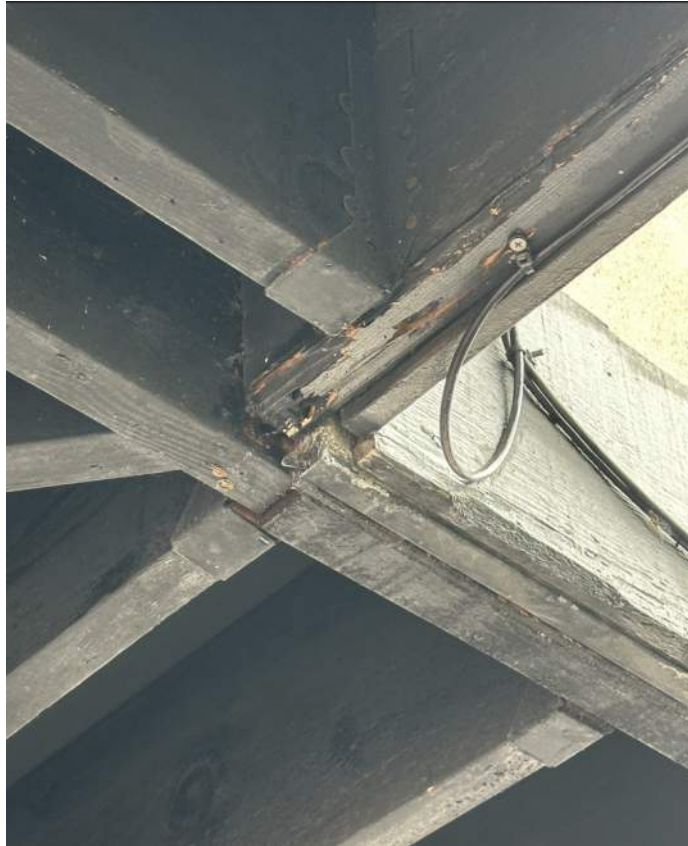
Figure 10- Dry Rot in Exposed Framing at Northmost Building
