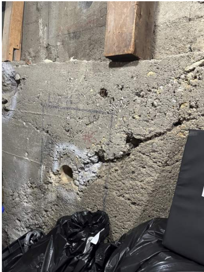
Figure 4- Void Vein in East Wall of Pre-1957 Structure
