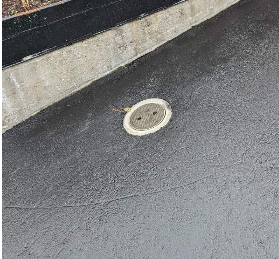
Figure 26 – Sanitary Sewer Cleanout
