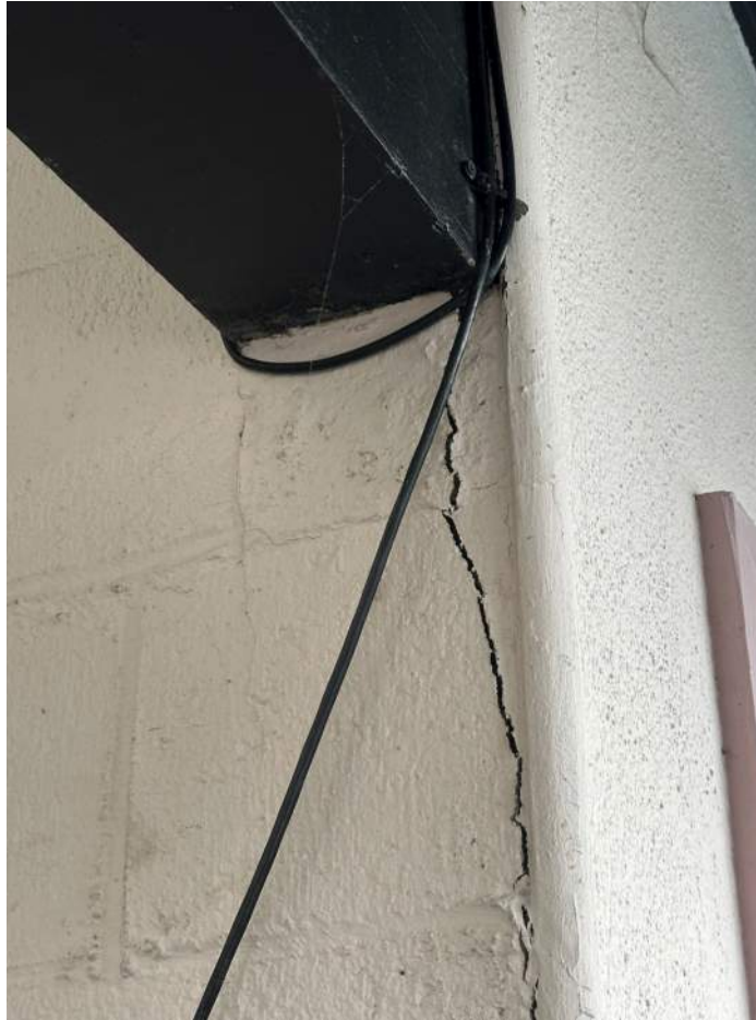
Figure 13- Fractured CMU Support Wall at Cantilevered 6x12
