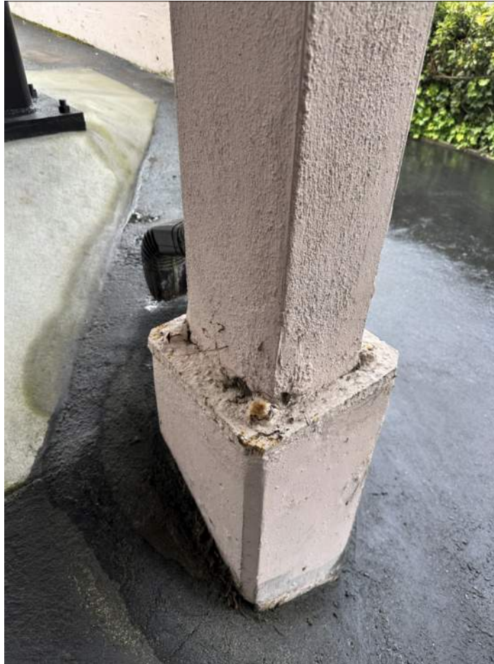
Figure 12- Corroded Base Plate and Anchors
