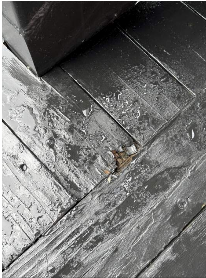
Figure 11- Dry Rot in Exposed Landing Framing at Northmost Building
