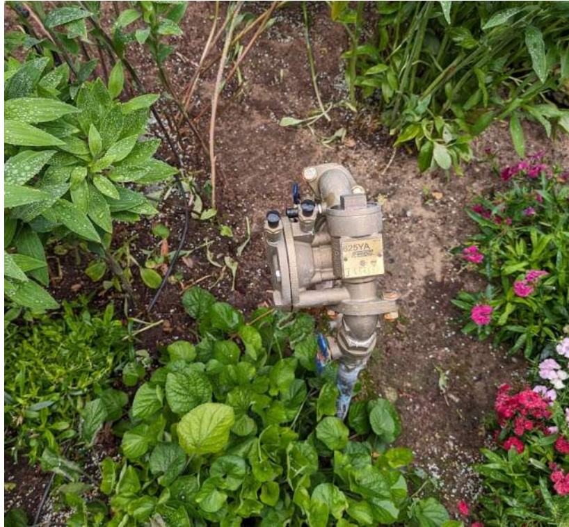
Figure 27 – Water Backflow Preventer
