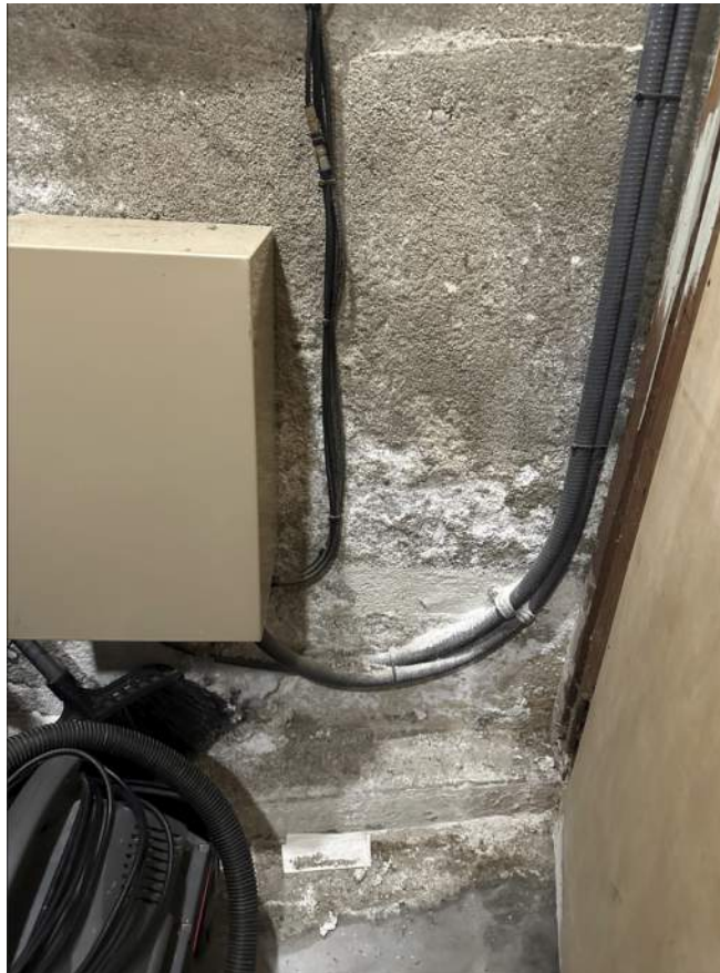
Figure 6- Efflorescence and Weak Concrete in South Wall of Pre-1957 Structure
