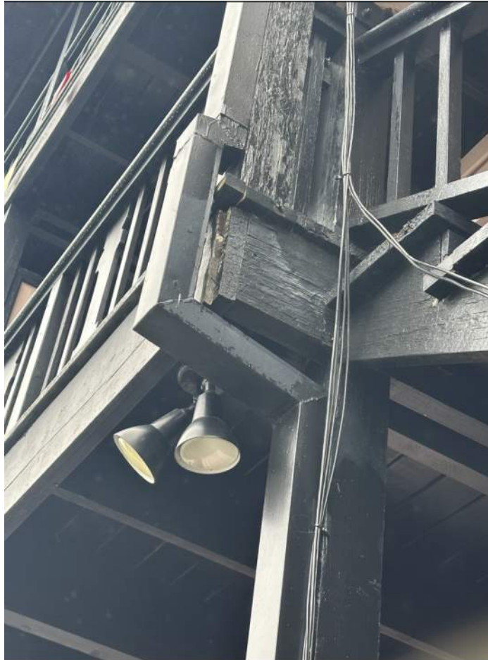
Figure 9- Example of Weathering in Exposed Framing
