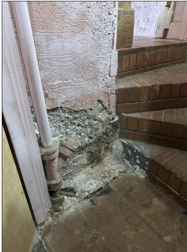
Figure 7- Additional Efflorescence and Weak Concrete in South Wall of Pre-1957 Structure
