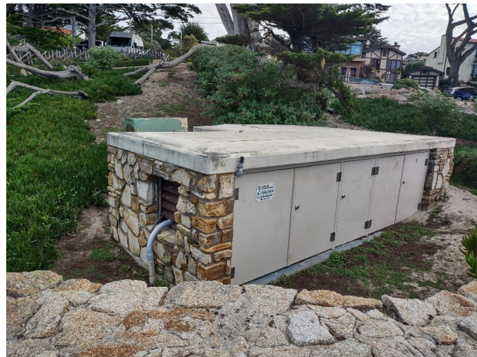
Wastewater lift station near 8 th Avenue
