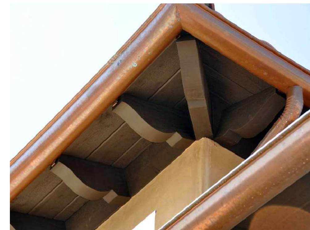
REDWOOD RAFTER TAILS AND T&G DECKING PAINTED TO MATCH WINDOWS AND DOORS GALVANIZED PAINTED HALF-ROUND GUTTERS WITH ROUND DOWNSPOUTS (BROWN COLOR TO MATCH RAFTER TAILS AND WINDOWS)
