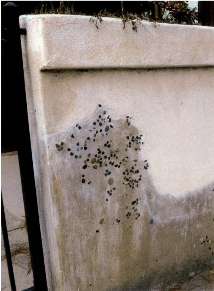
Figure 6a. Photos from application materials submitted with DR 13-24 (Photo 1). Photo is a of the northern most portion of the wall fronting Dolores Street where the wall connects to a steel gate (see Figure 5, above). Wall has been installed with a planter, a lip has been added to the top area around the planter, and the wall appears to have been partially plastered over.
