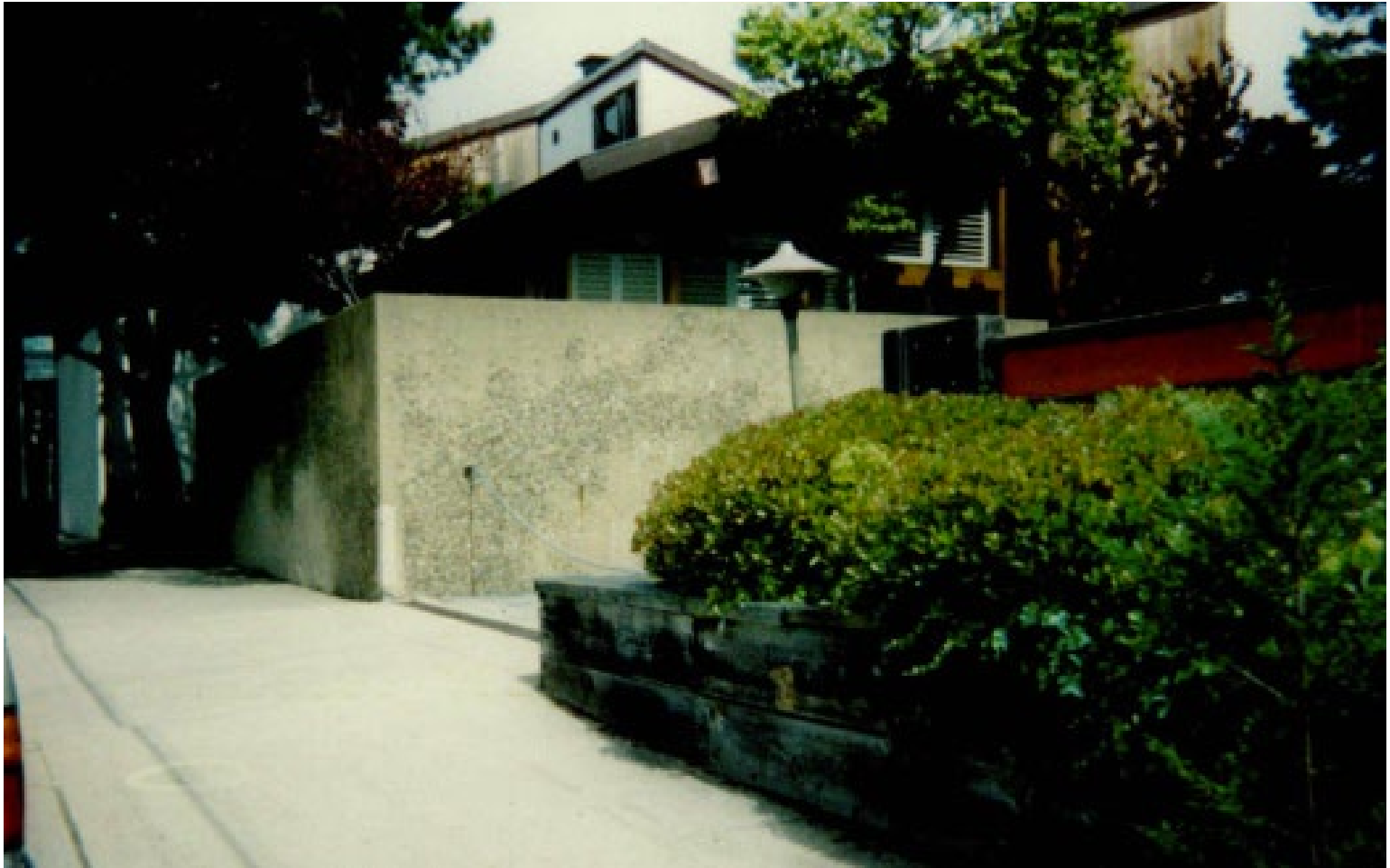
Figure 3a. Photo of original concrete wall submitted as part of application materials for DR 99-35.
