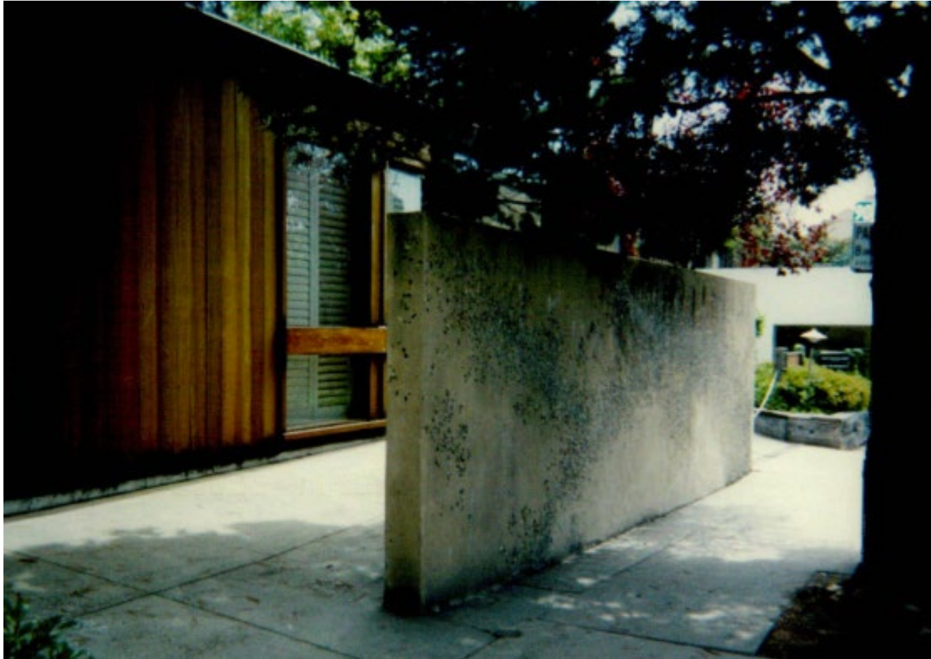
Figure 3c. Photo of original concrete wall submitted as part of application materials for DR 99-35.
