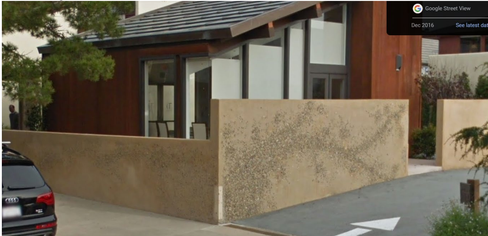
Figure 8. Wall viewed from Dolores Street. December 2016. Wall on fronting Dolores is repaired. All wall portions appear to be painted or stained from previous condition (see Figures 3, 5, and 6)
