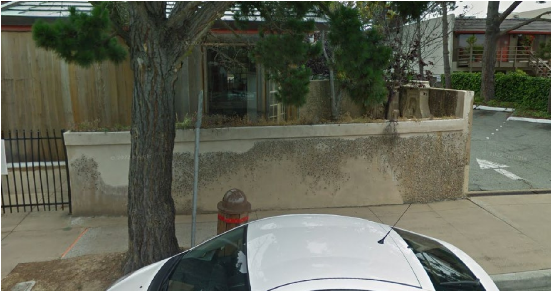
Figure 5. Wall viewed from Dolores Street. June 2011. Image shows wall had been cut down on Dolores Street Elevation with planter on top. Portion of wall returning to Community Room visible beyond.
