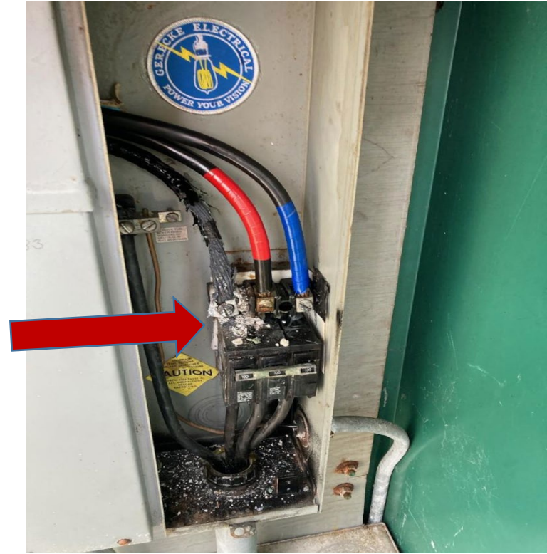
North Lot Electrical Panel
